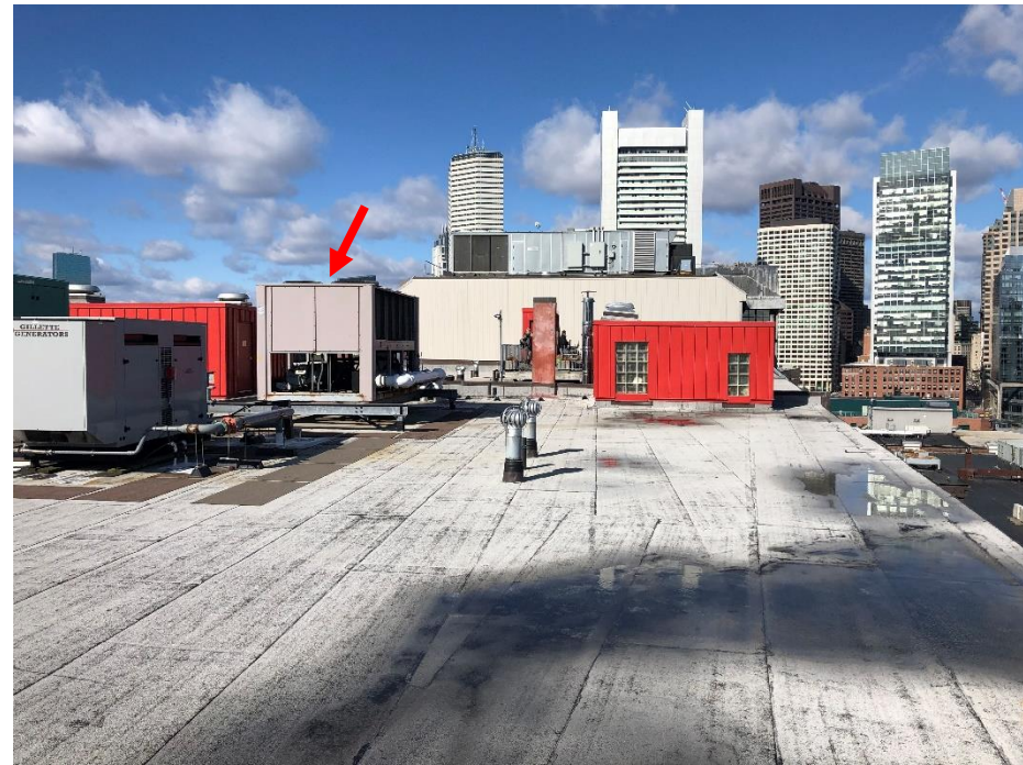
Looking west (chiller noted with red arrow)
