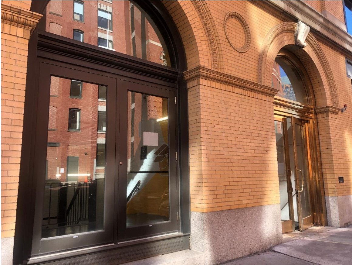
Exterior, brass clad main entry doors shown at right Existing grey metal clad stairwell doors shown at left
