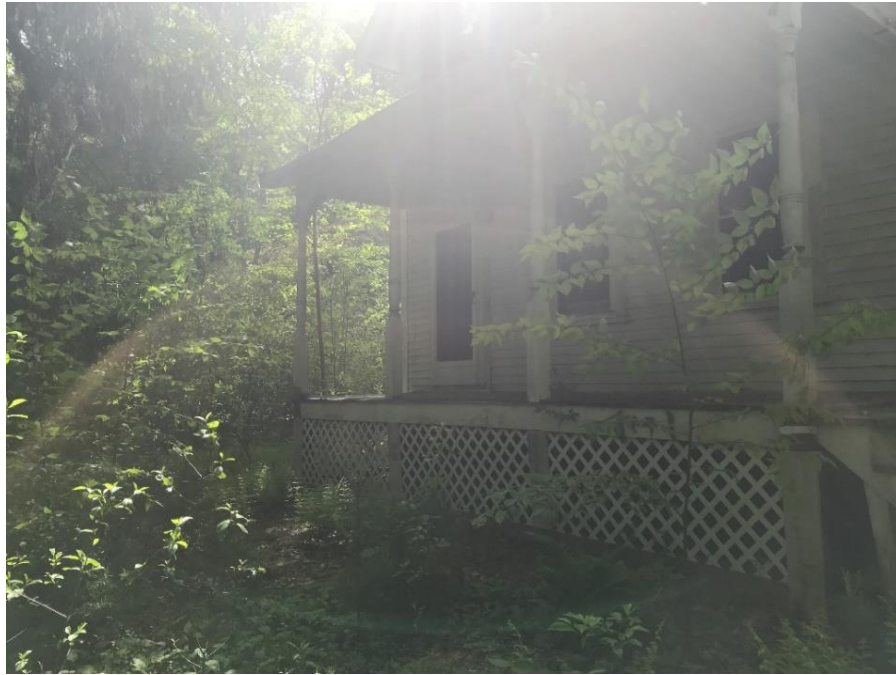
Photograph 4: View (looking west) of the existing elevated porch located on the east side of residence to be removed.
