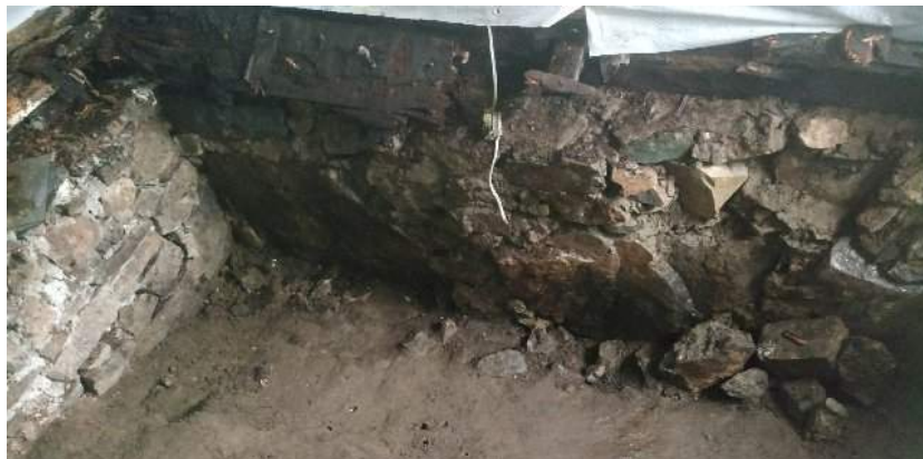
Figure 1- Floor boards were completely removed in the porch area
