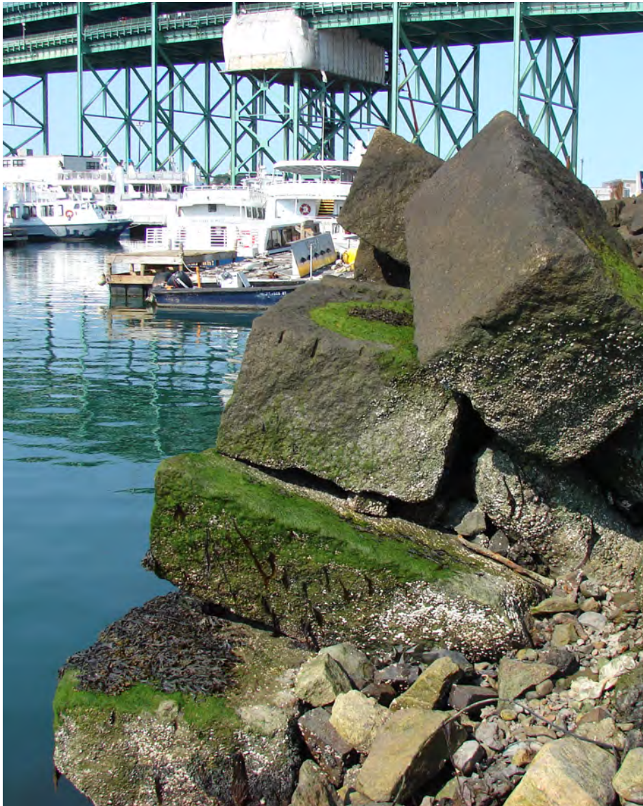
Photo 3: Collapsed granite block seawall
