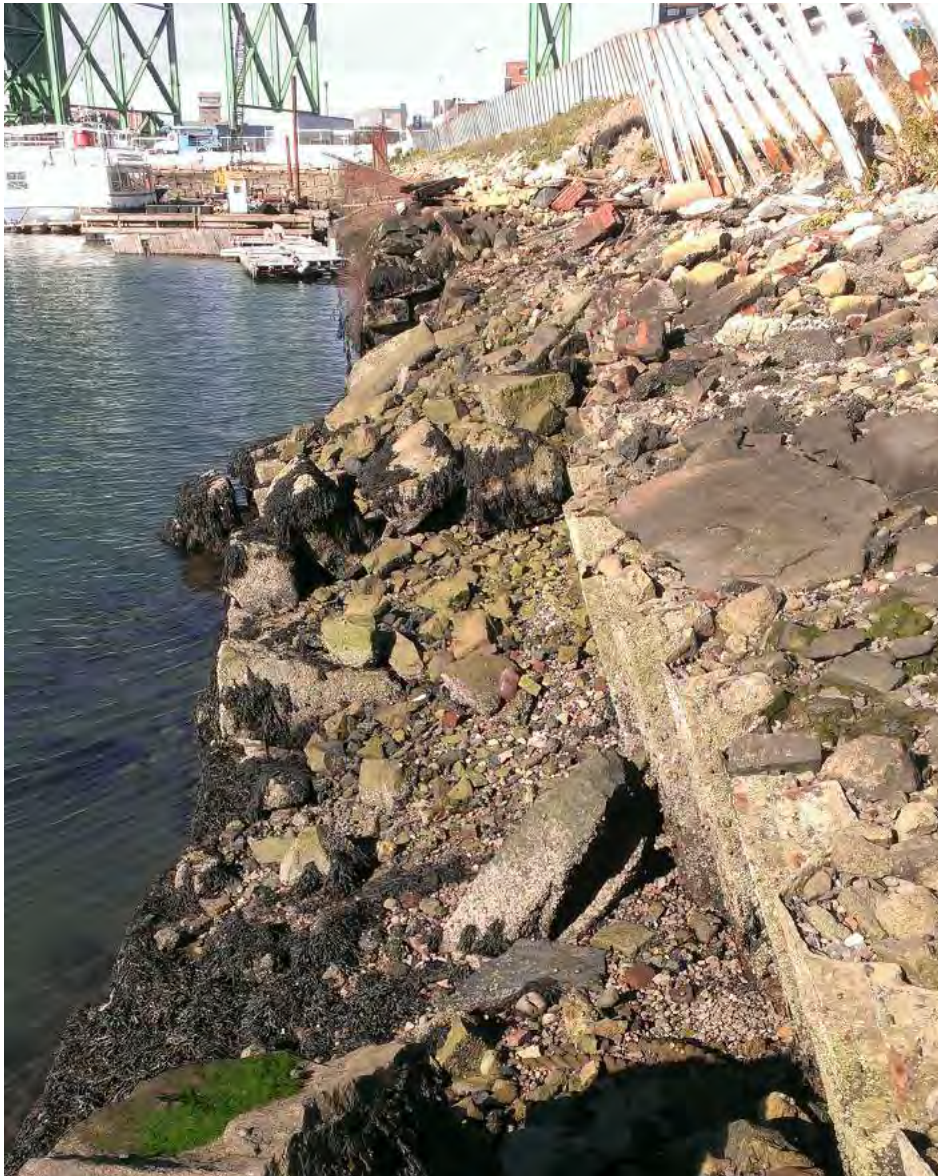
Photo 5: Failed seawall looking west
