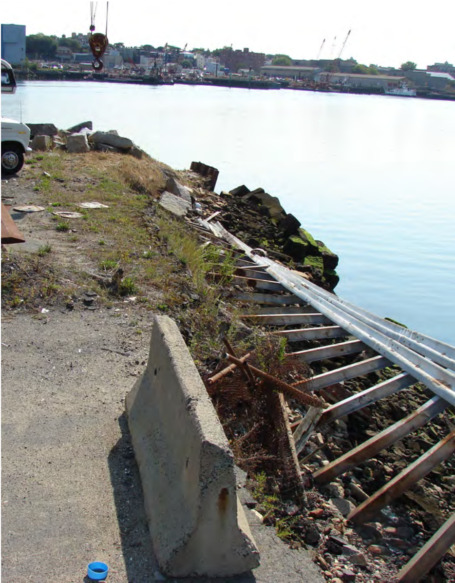
Photo 1: Failed seawall facing east
