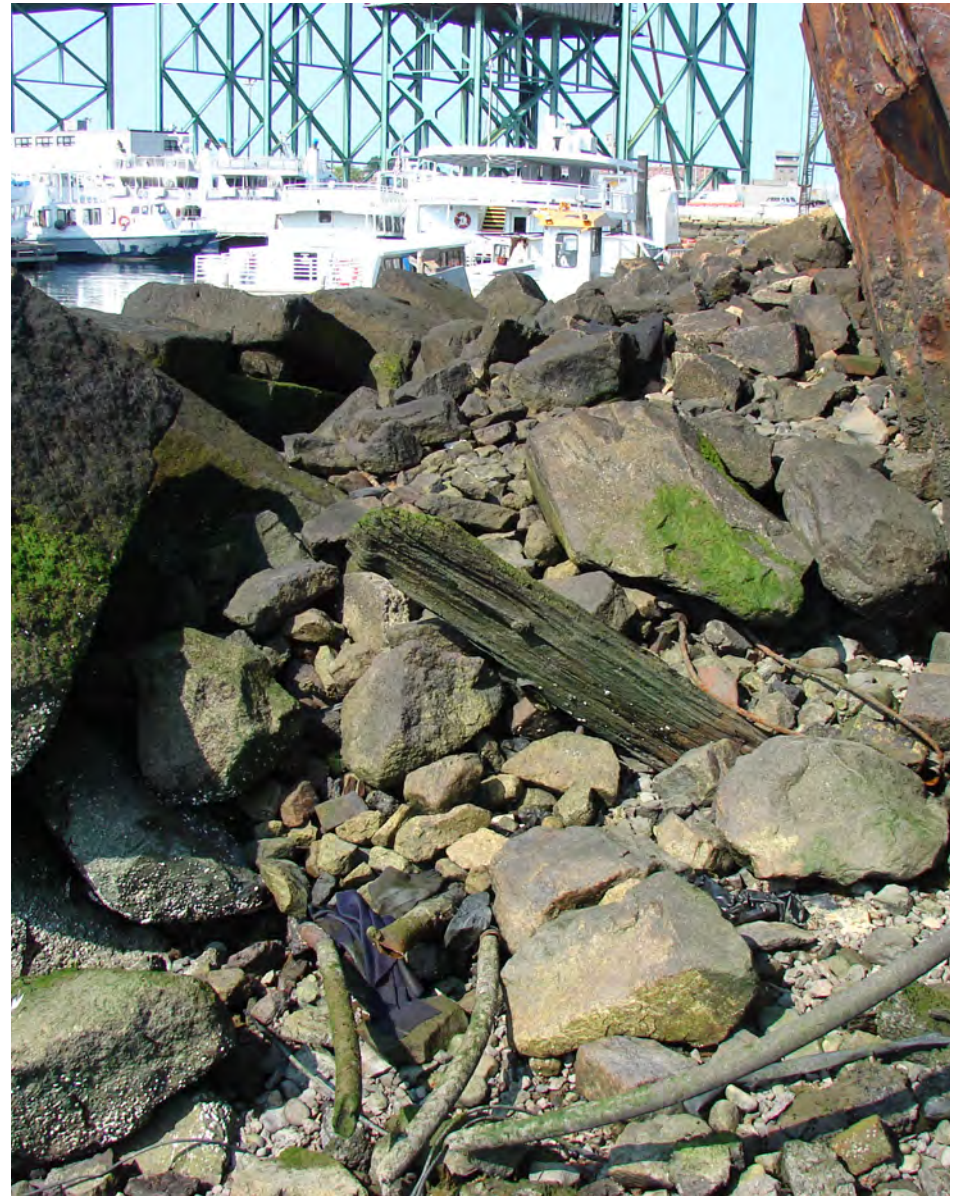
Photo 2: Failed seawall facing west
