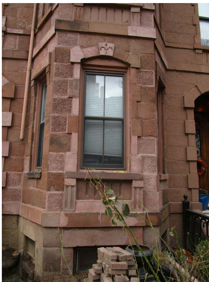
Discolored Existing Masonry Detail
