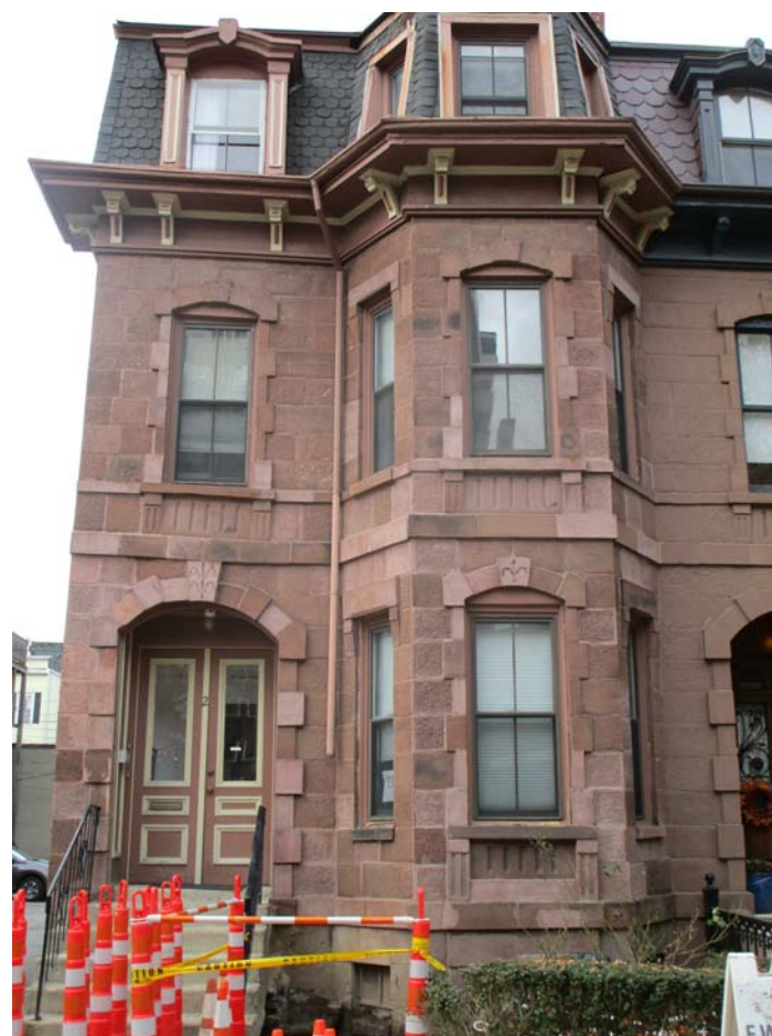
Discolored Existing Masonry
