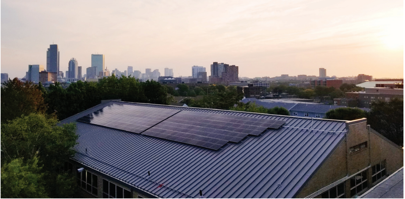
The City of Boston has installed solar panels on the roof of the Tobin Community Center.
