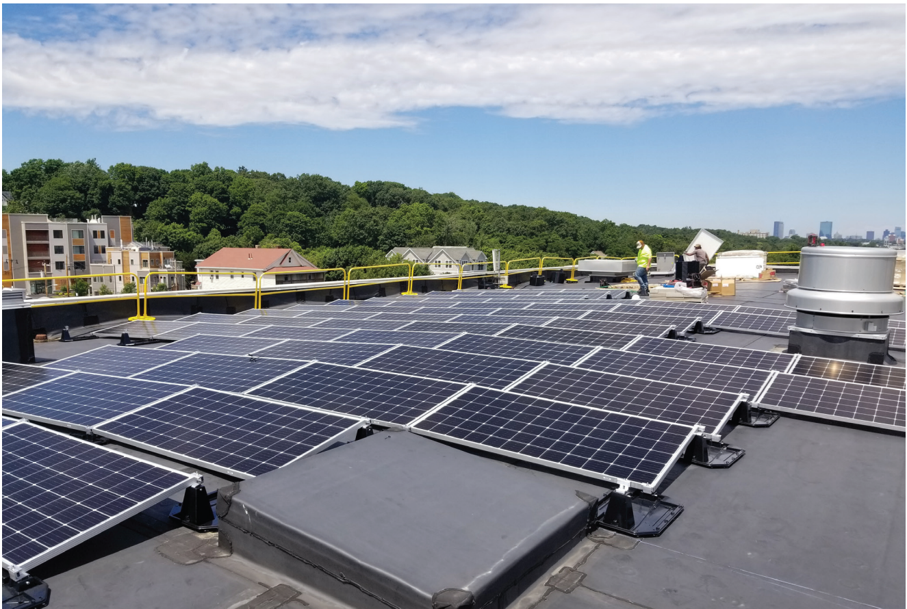
The City of Boston has installed solar panels on the roof of the Roslindale Community Center through the Renew Boston Trust program.
