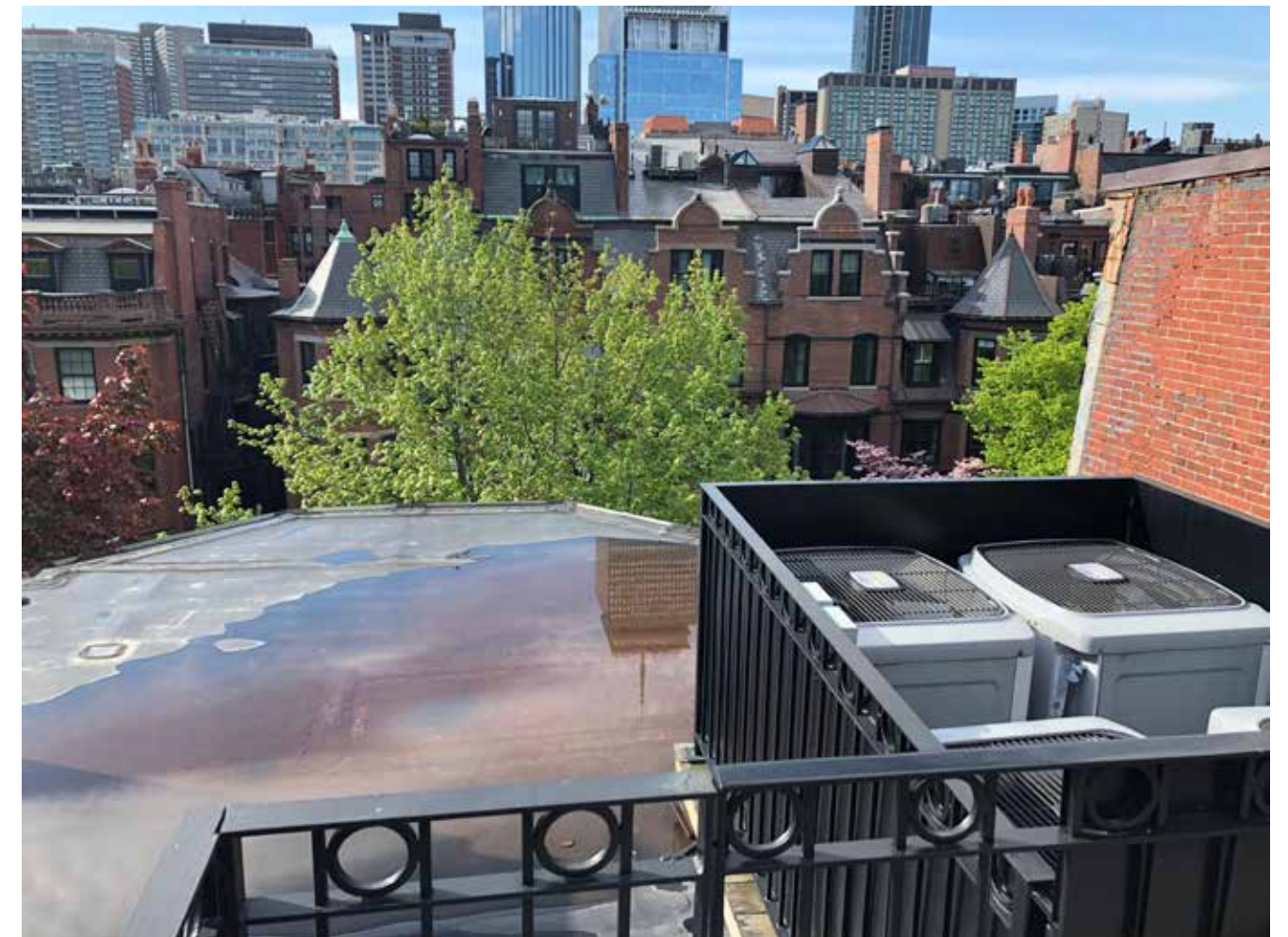
Mechanical Equipment - Existing Conditions
