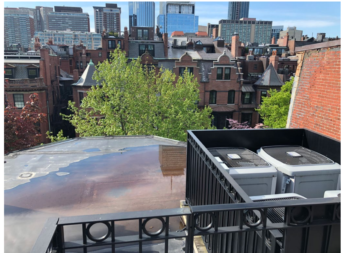
Mechanical Equipment - Existing Conditions
