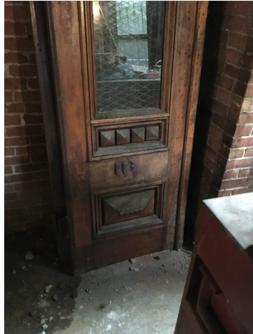
PROPOSED DOORS FOR 11HF CLAREMONT PARK (ONE OF PAIR SHOWN) (RE-USED FROM INNER VESTIBULE)
