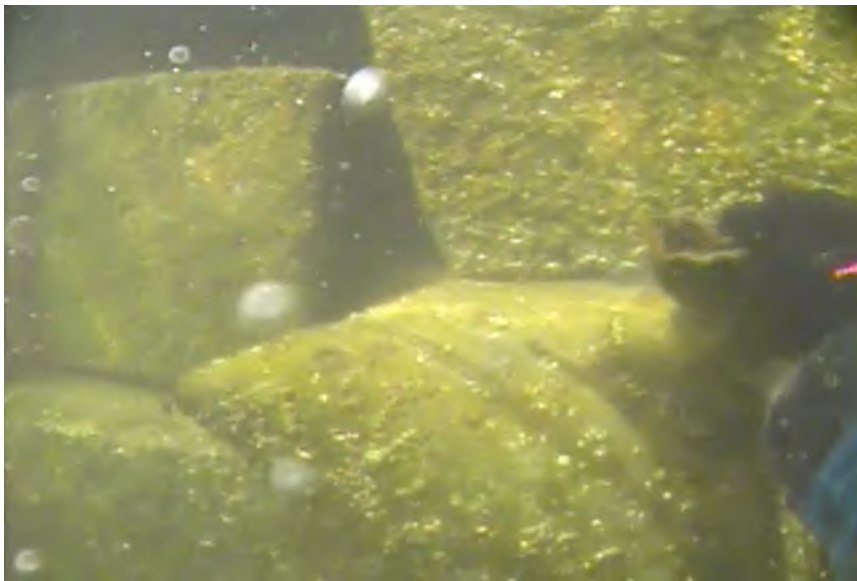
Typical Displaced Granite Blocks in Proposed Repair Area
