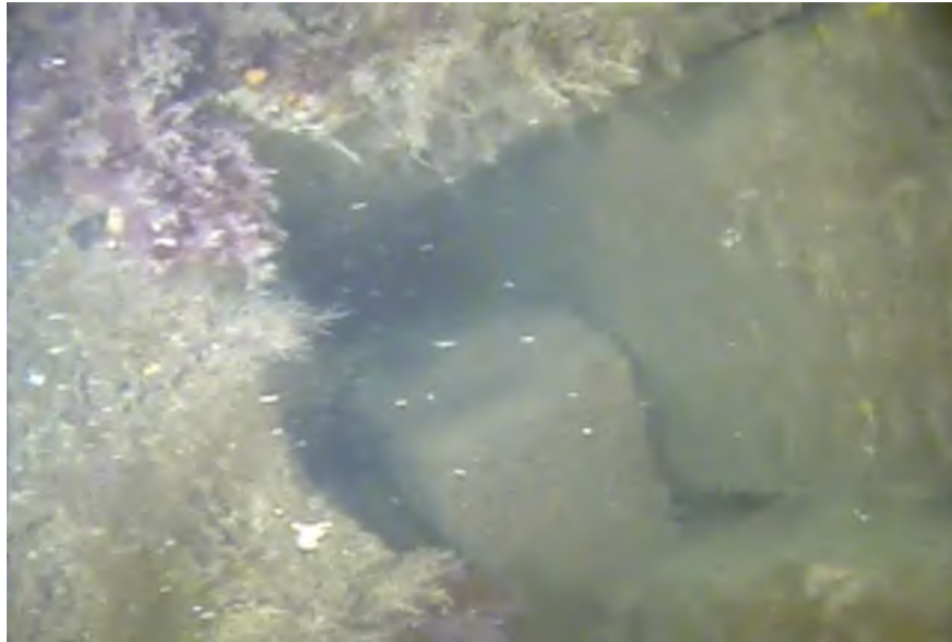
Typical Seawall Voids in Proposed Repair Area
