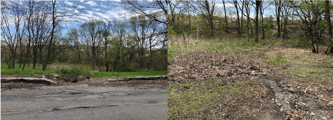
Photo 9. Views of the location where stormwater runoff from South Street flows into Bussey Brook Meadow. Erosion and sedimentation has impacted the existing slope and meadow.
