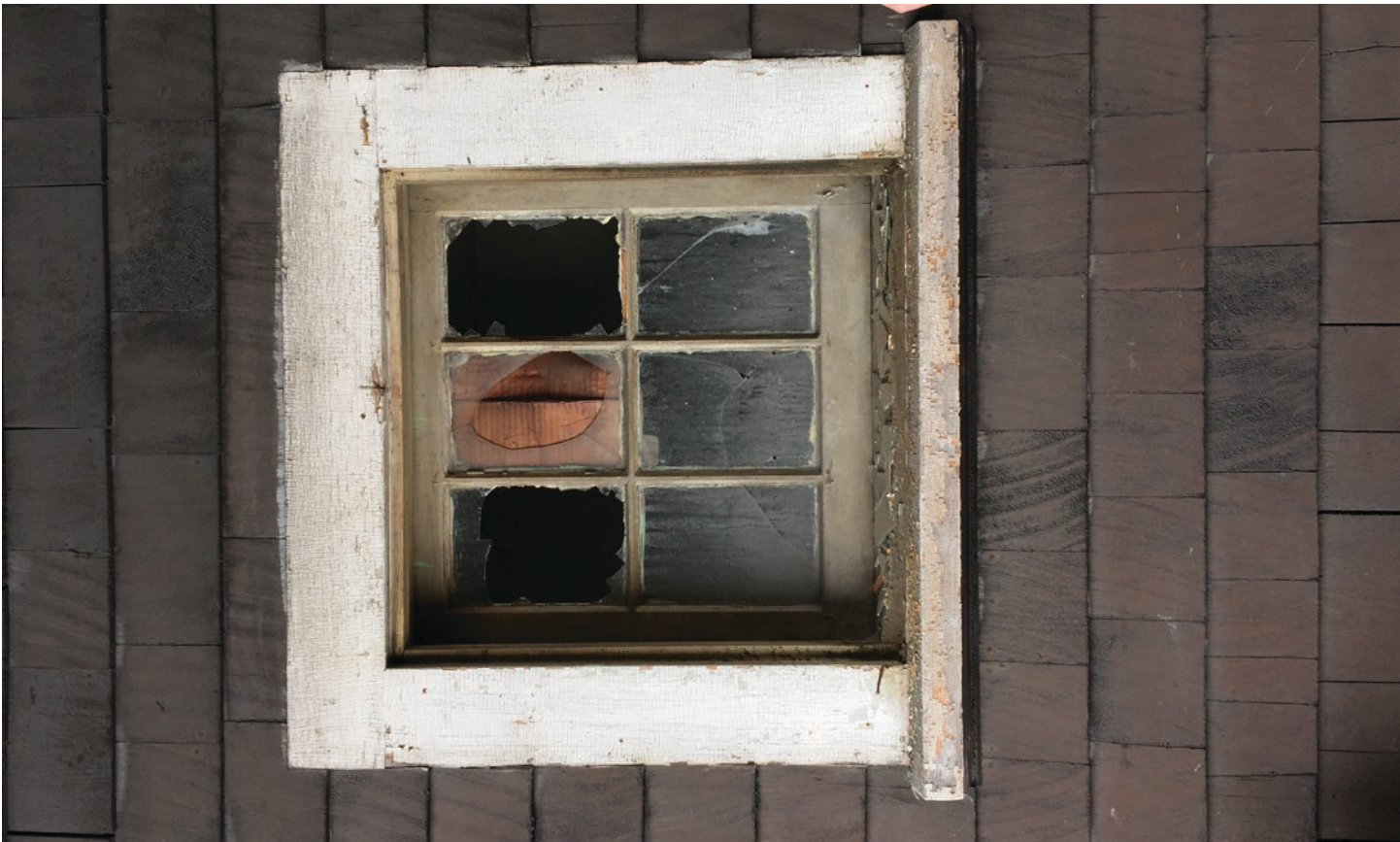
Figure 39: Building D Hopper Window
