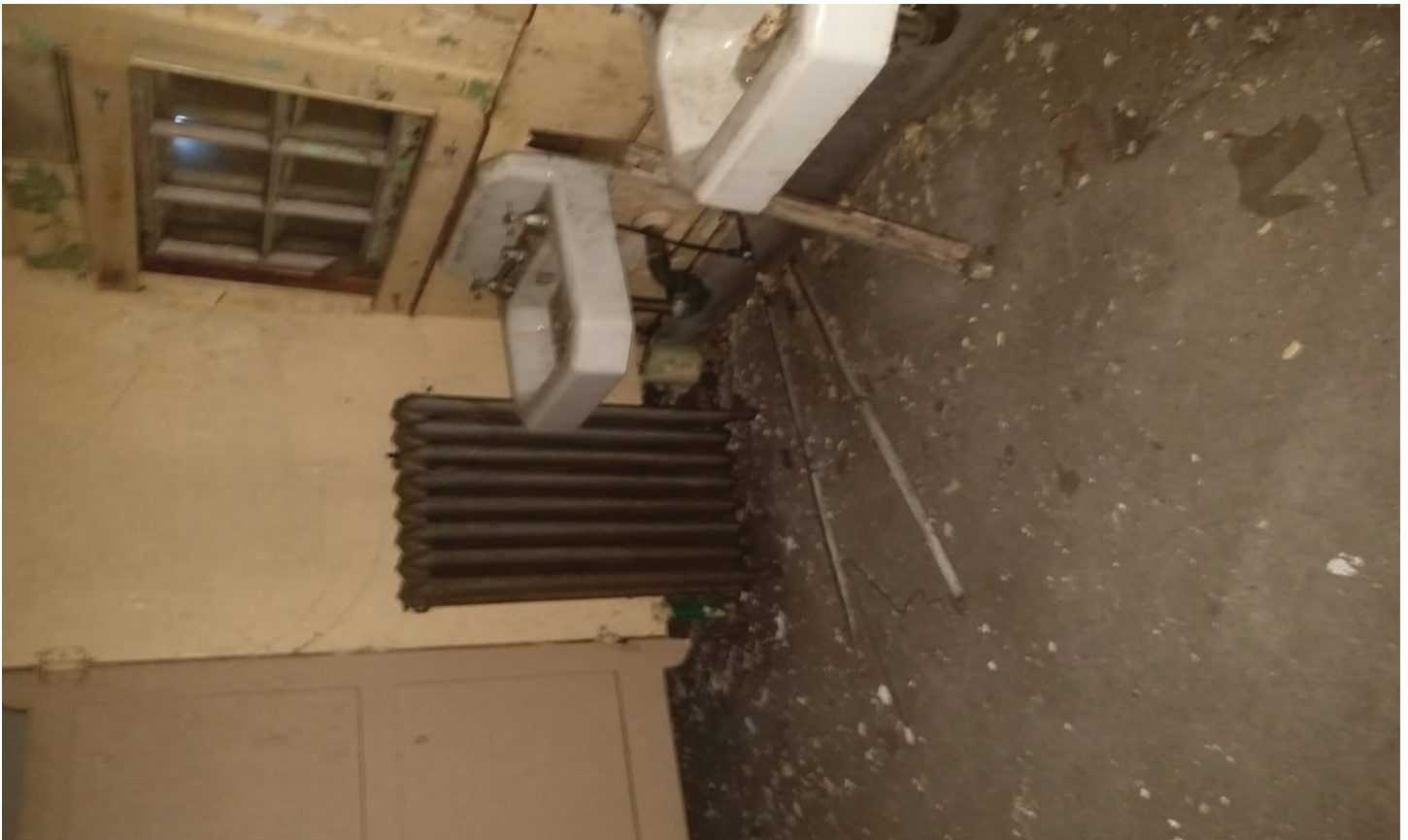
Figure 82: Building H Interior 2nd Floor Fixtures
