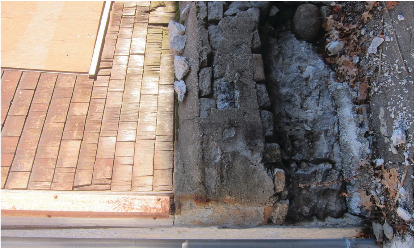
Figure 12: Building C Foundation Deterioration
