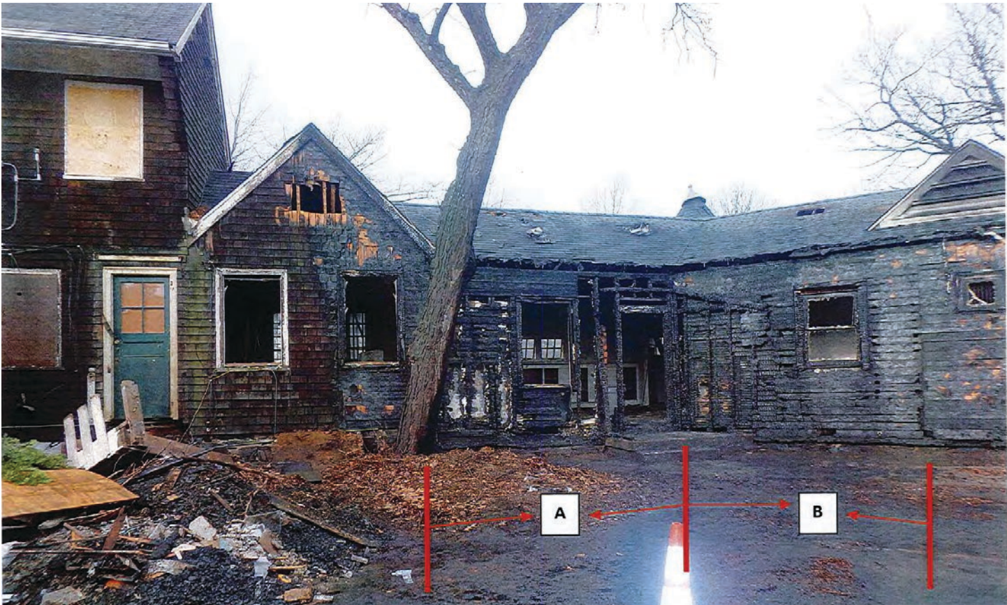
Figure 33: Building G Courtyard Entry Fire Damage
