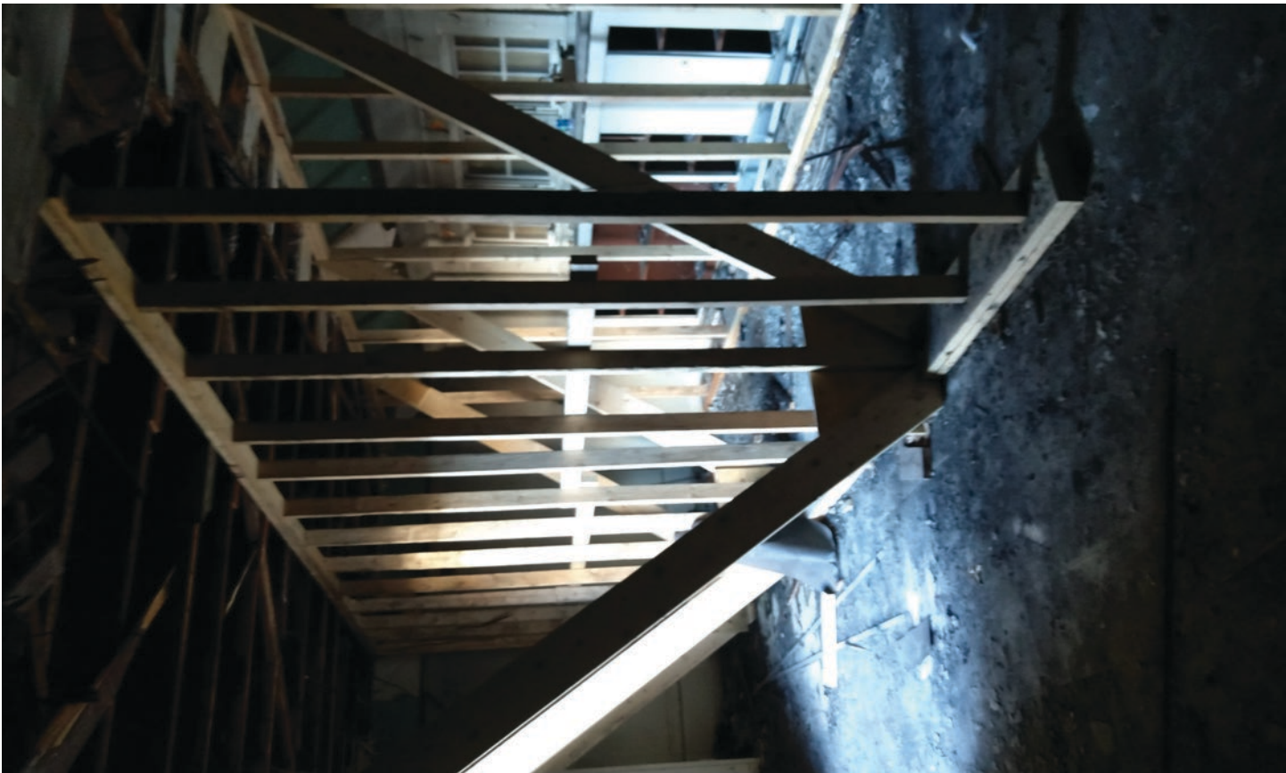
Figure 76: Building G Interior at Fire Damage
