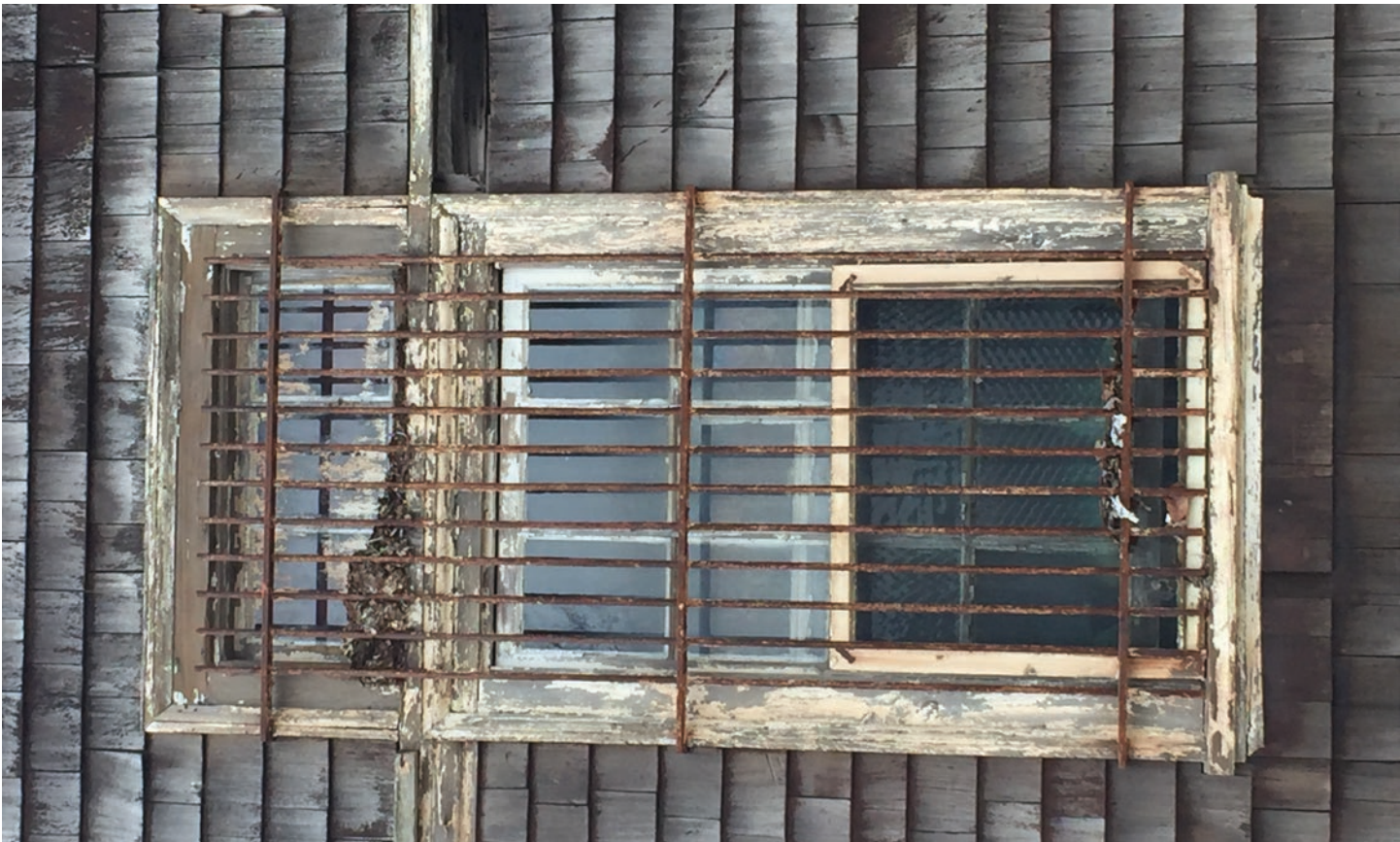
Figure 47: Building H Barred Window at Jail
