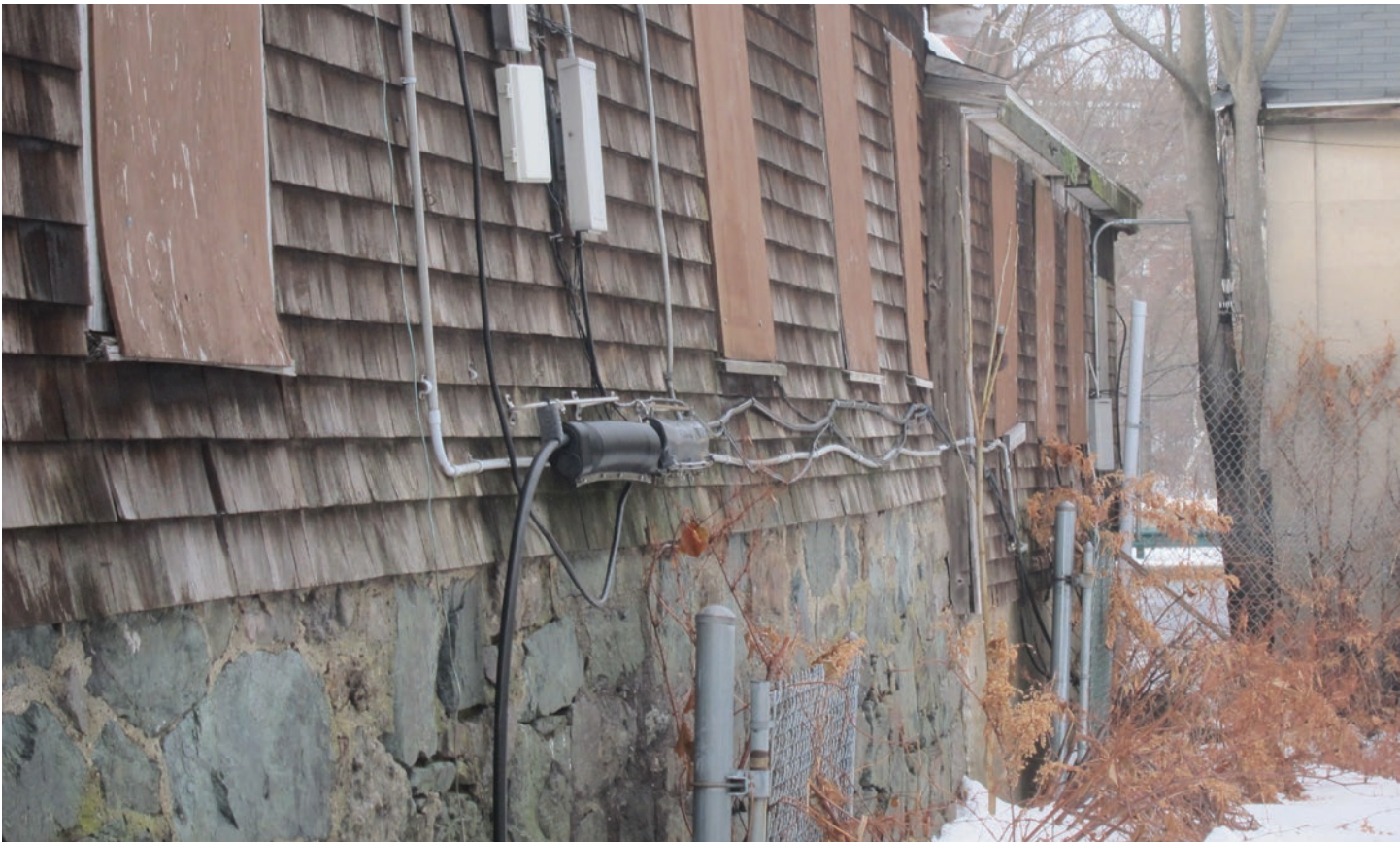
Figure 13: Building D Foundation Bulge
