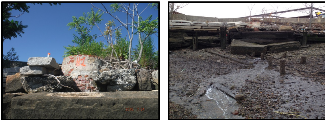
Figure 2-10. Outfall H showing (l) TMH H1 with granite block retaining wall and (r) water flowing below collapsed granite retaining wall blocks.
