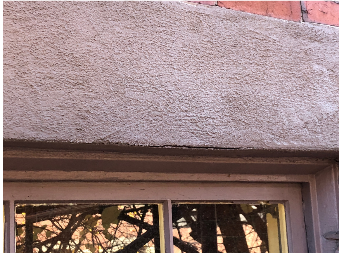
CRACKED STUCCO @ LINTEL
