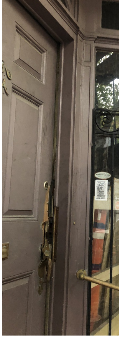
EXISTING ENTRY DOOR DAMAGED AT HANDLE
