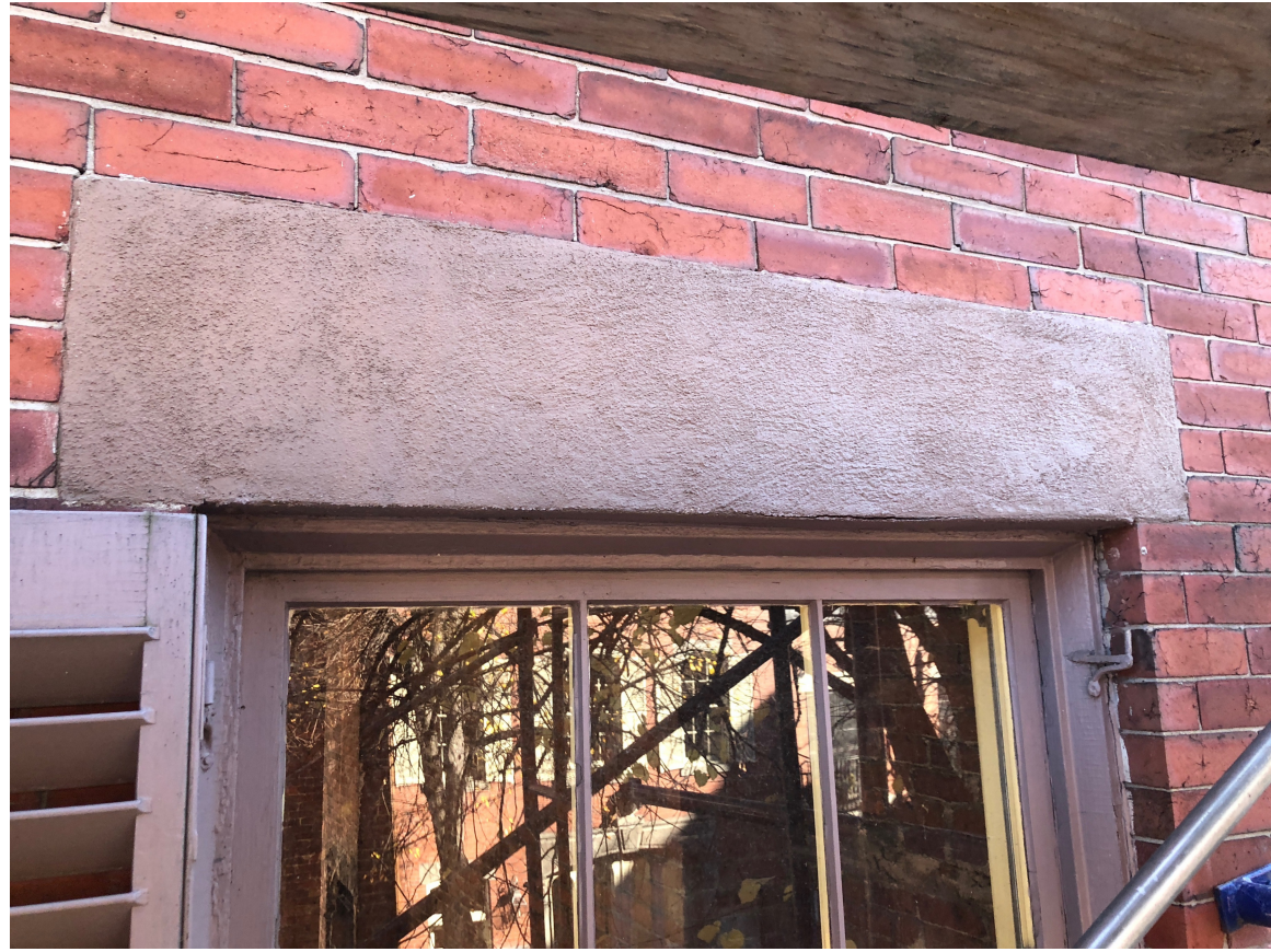
CRACKED STUCCO @ LINTEL
