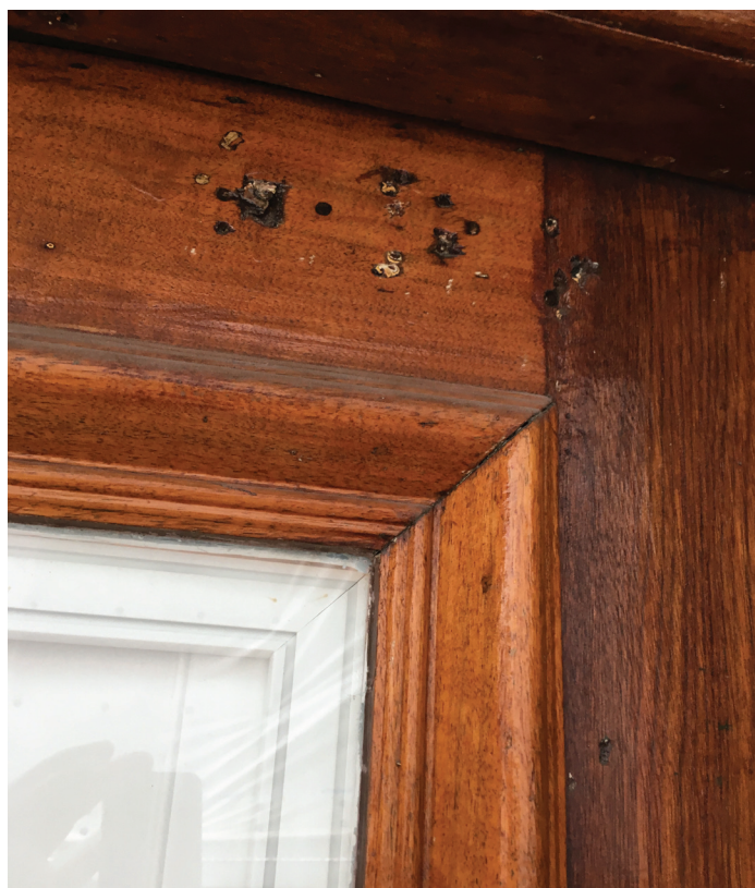
damage from old closer
