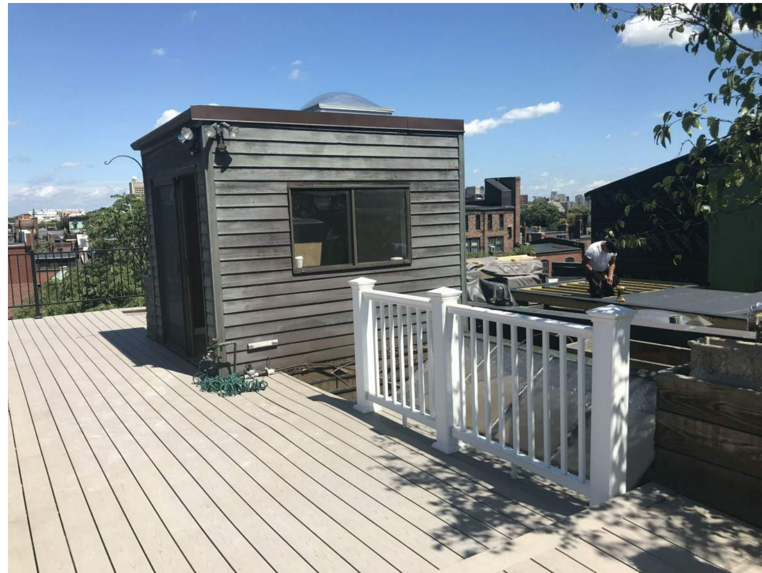
EXISTING HEAD HOUSE - 327 COMMONWEALTH AVE NEW HEAD HOUSE AND ROOF DECK UNDER CONSTRUCTION - 329 COMMONWEALTH AVE (RIGHT SIDE OF PHOTO)
