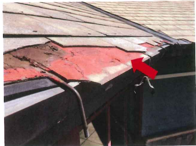
View of the broken and displaced gutter at the west side of the roof. Broken, cracked, loose, and missing shingles were noted throughout the various roof areas.
