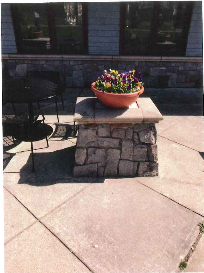
Detail of support pillars (that no longer are needed) and failing concrete paving.
