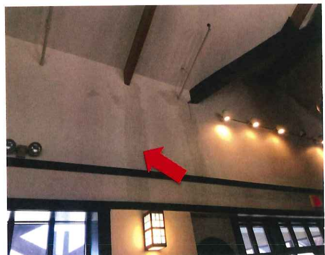
Water staining at the upper wall locations
