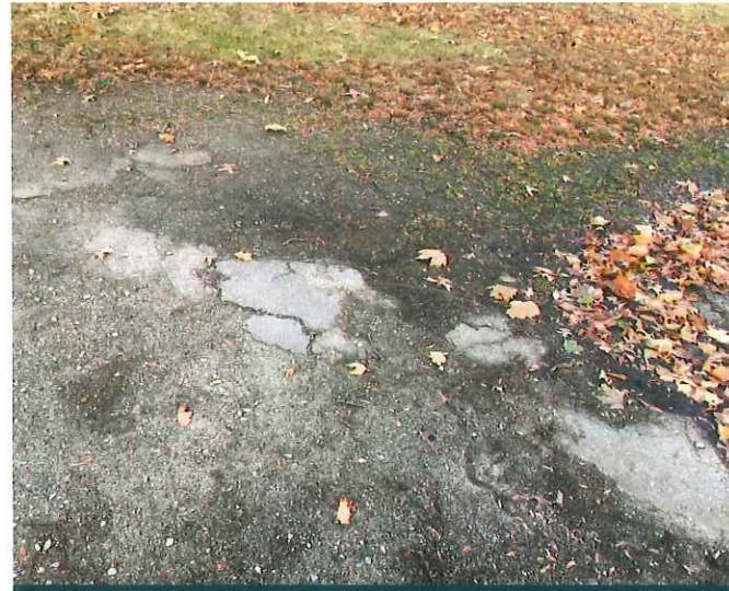
Abandoned asphalt should be fully excavated
