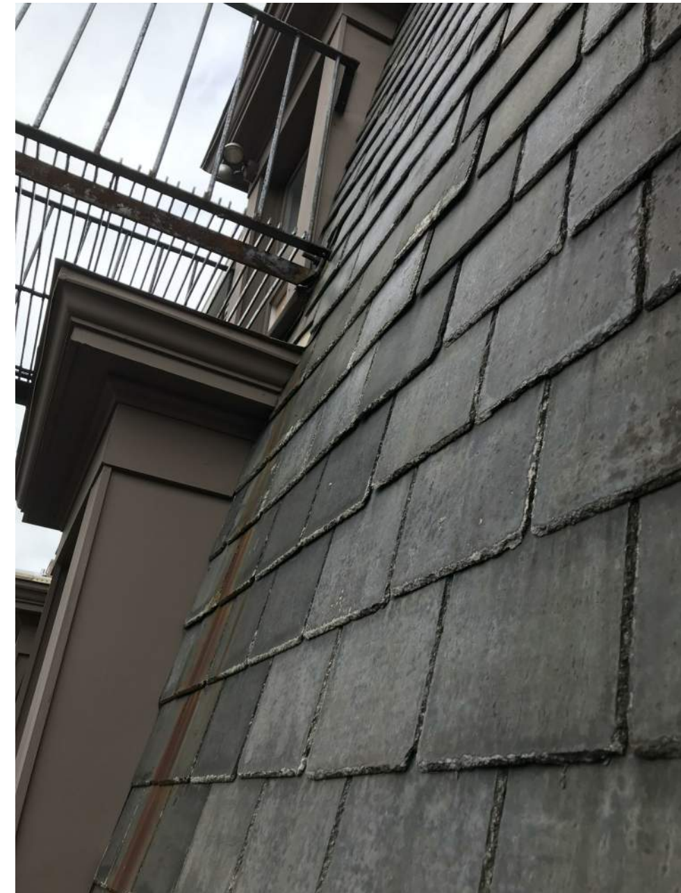
ROOFING TO BE REPAIRED AND RESTORED AS REQUIRED.
