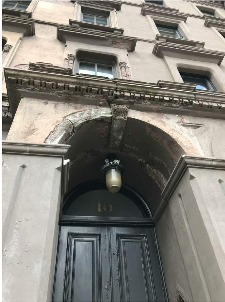
REPAIR AND RESTORE EXISTING STONE STOOP, PAINT HC-69 REPAIR AND RESTORE FRONT DOOR. REPLACE EXISTING PENDANT.
