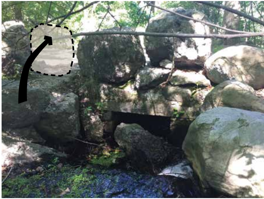
Restore fallen edge stones (stones have fallen down to the brook bank)
