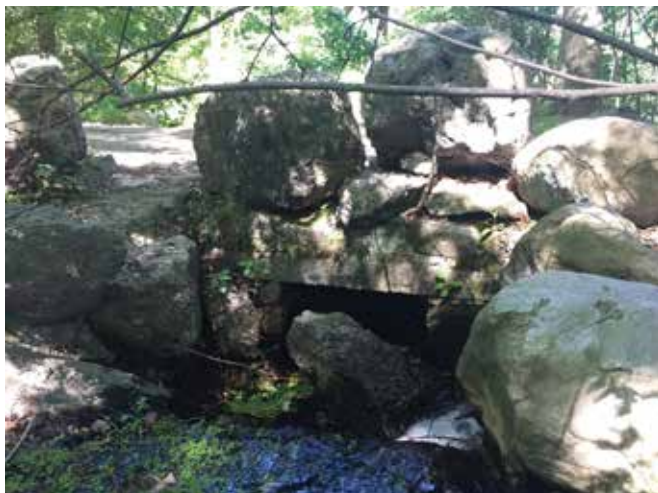
Missing edge stones (standing on Sping Pond bank)
