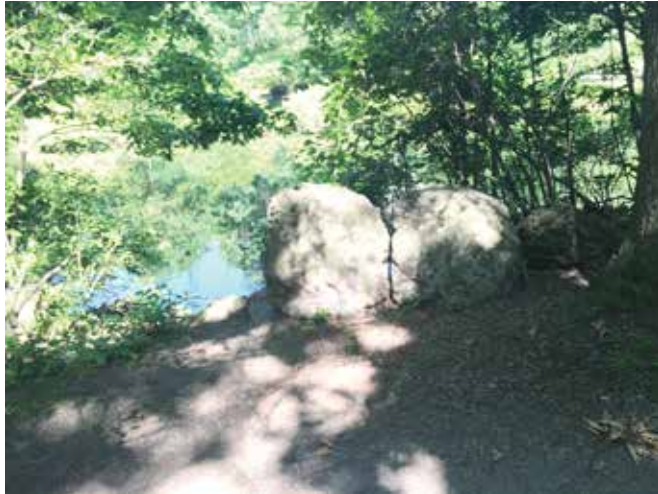
Missing edge stones (standing on bridge)
