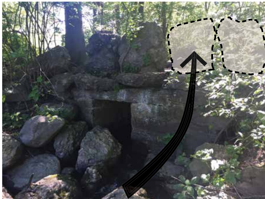
Restore fallen edge stones (stones have fallen down to the pond bank)
