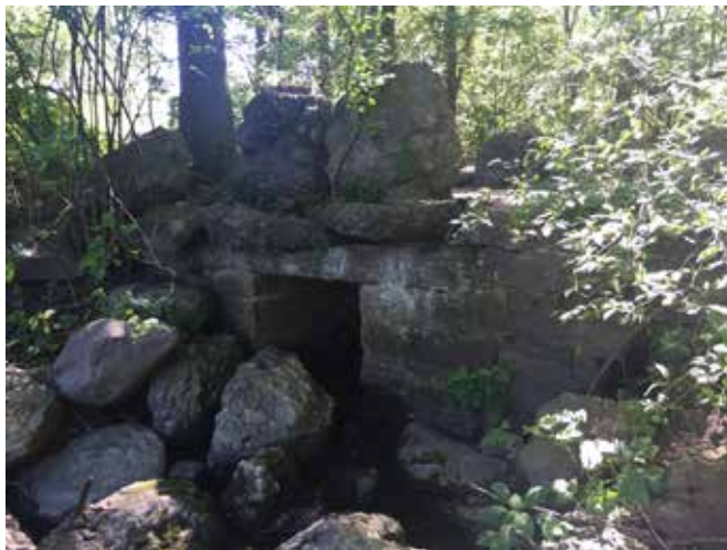
Missing edge stones (standing on Willow Pond bank)
