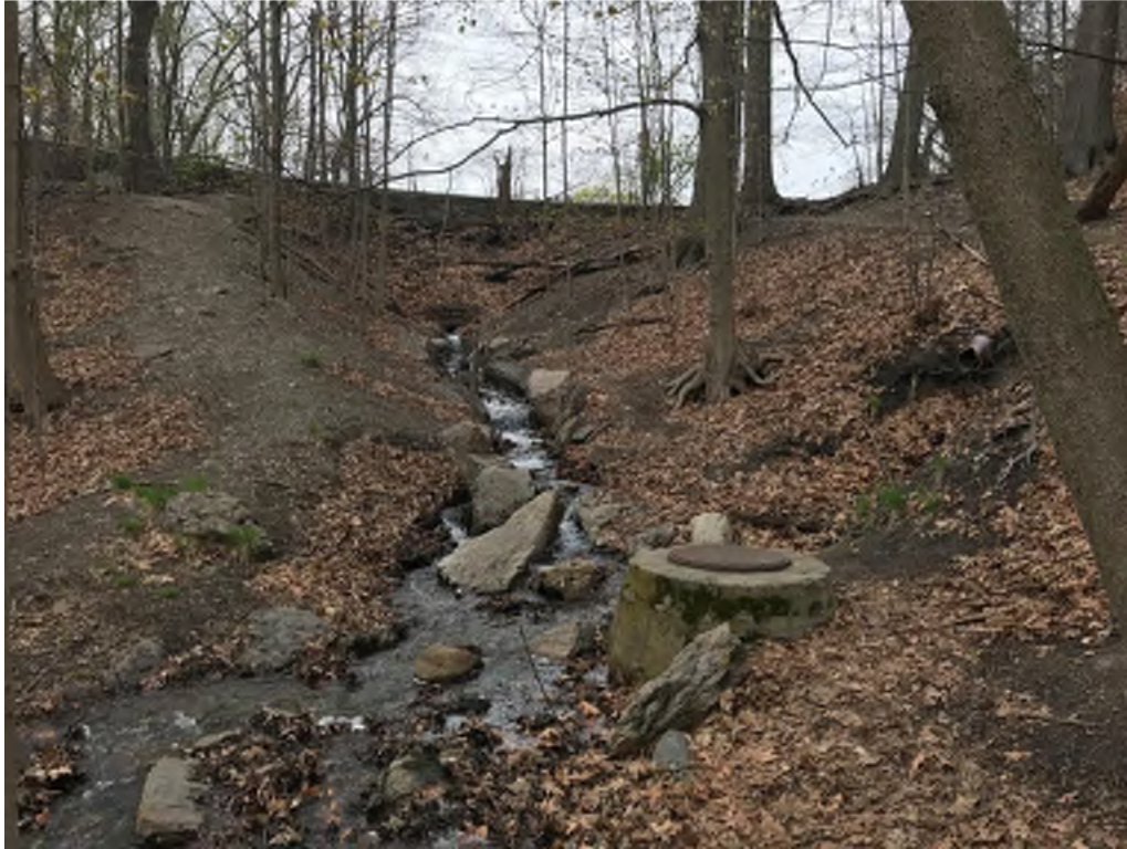
Photo 1: Overflow from the pipe system between Jamaica Pond and Wards Pond
