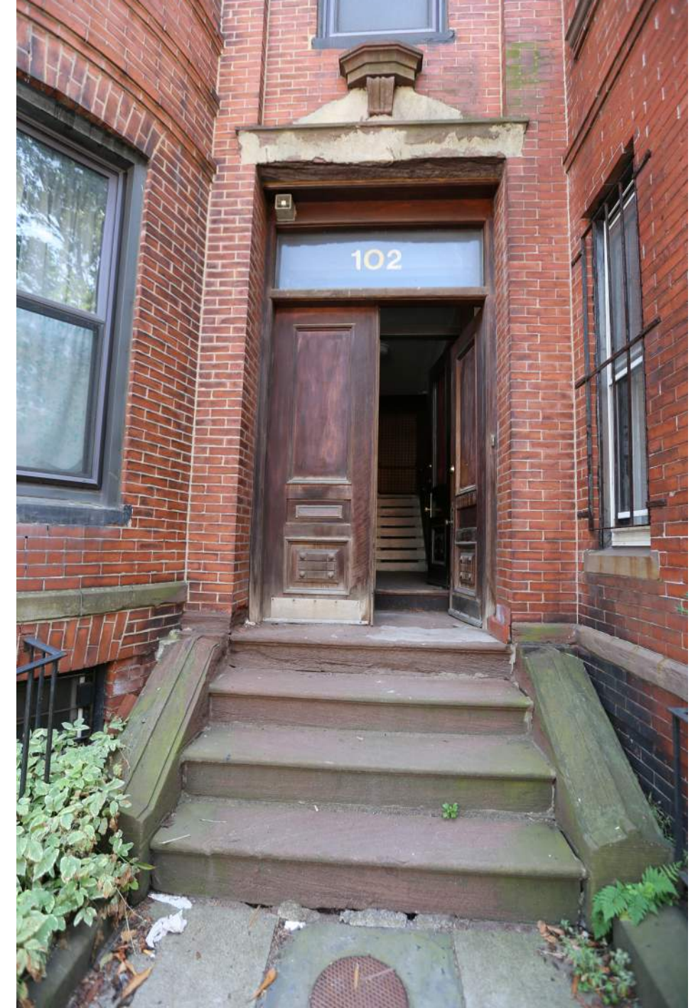
EXISTING STOOP AND BROWNSTONE ORNAMENT TO BE REPAIRED AND RESTORED. EXISTING WOOD DOORS TO BE REPAIRED AND RESTORED.
