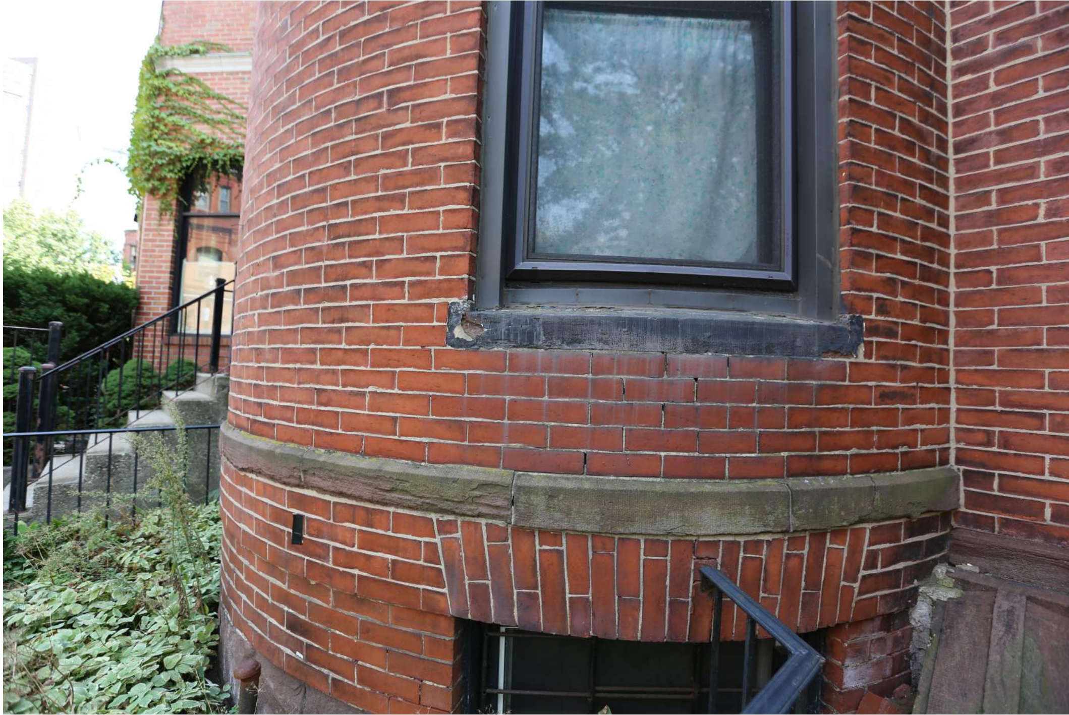
LINTELS TO BE REPAIRED AND RESTORED. NON-ORIGINAL WINDOWS TO BE REPLACED WITH '2 OVER 2' WOOD WINDOWS. MASONRY TO BE REPAIRED AND REPOINTED TO MATCH EXISTING.
