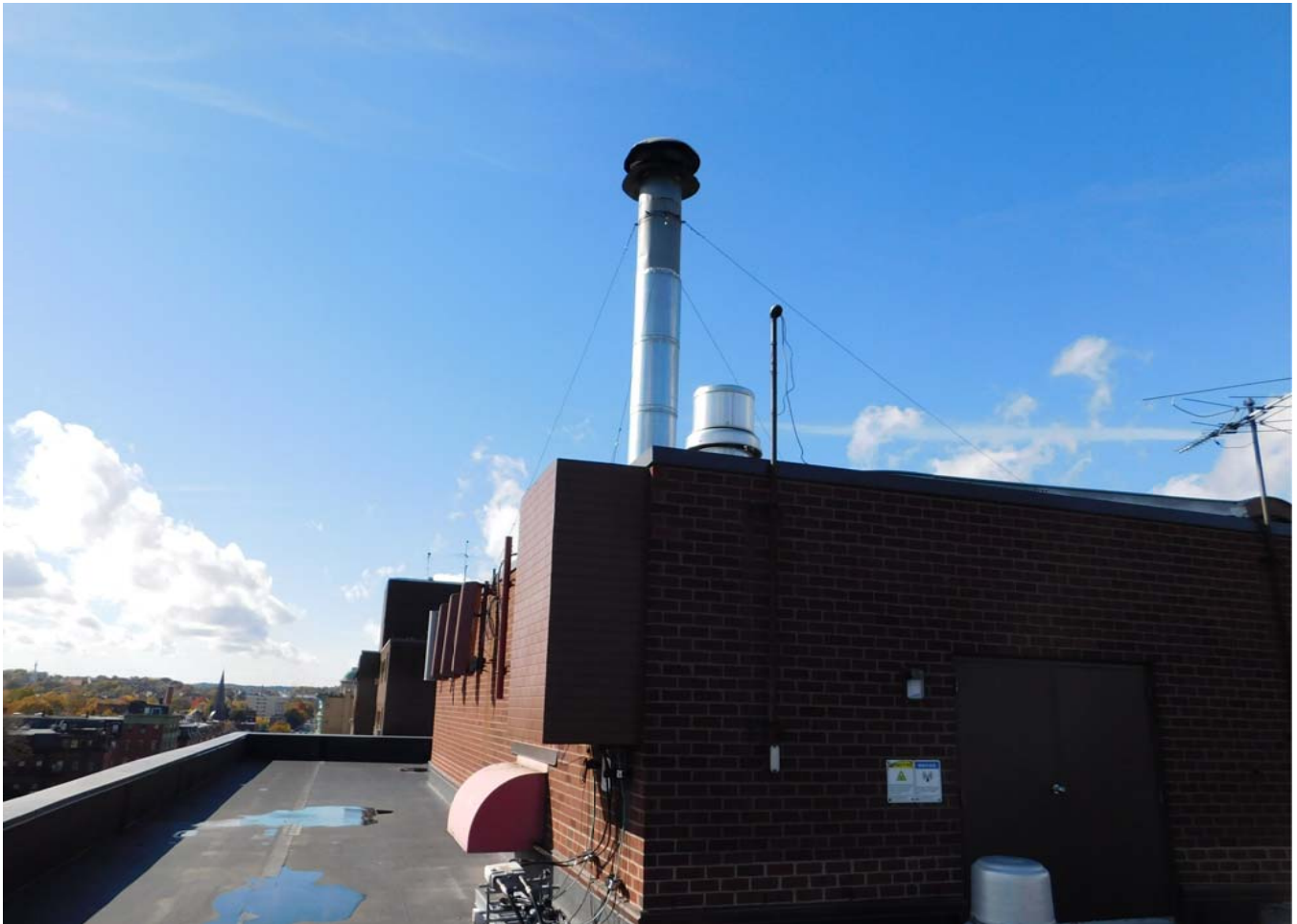
Existing Beta Sector Antenna RF Enclosure
