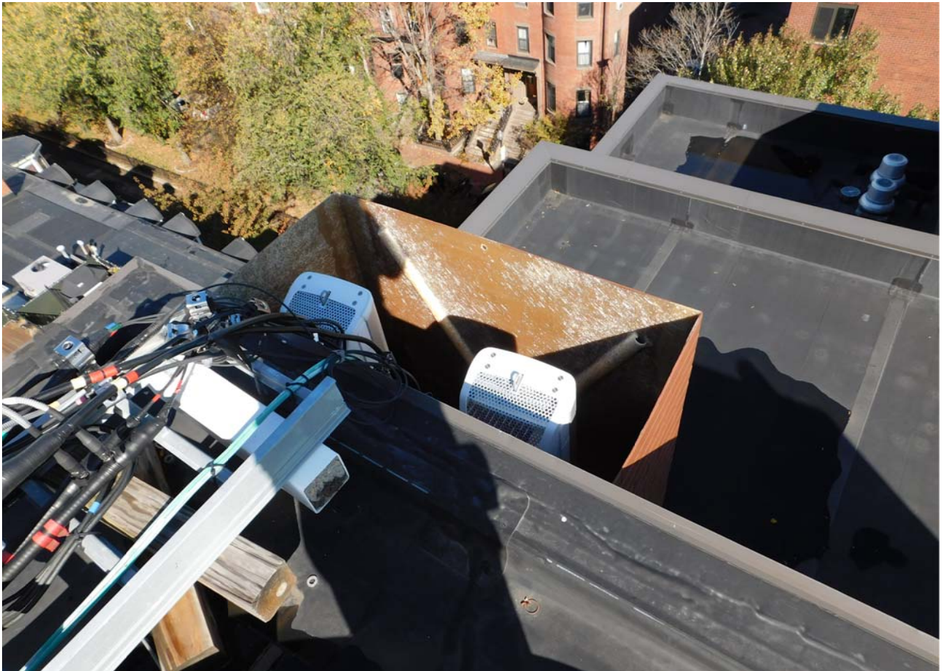
Existing Alpha Sector Antennas - Top View
