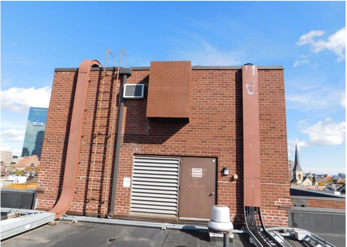
Existing Gamma Sector Antenna RF Enclosure
