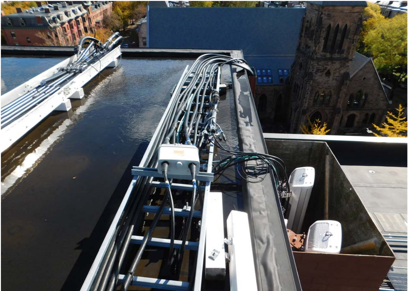
Existing Gamma Sector Antennas - Top View
