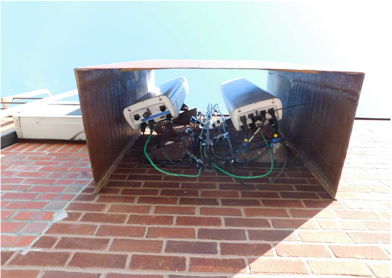
Existing Gamma Sector Antennas
