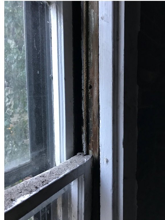
POSSIBLE ORIGINAL SASH AND FRAME IN DISREPAIR
