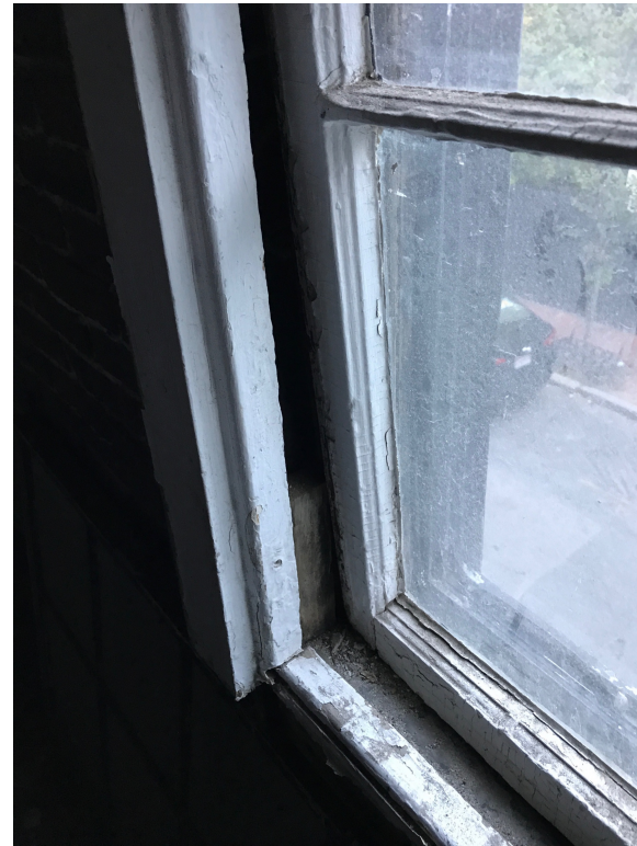
POSSIBLE ORIGINAL SASH AND FRAME IN DISREPAIR
