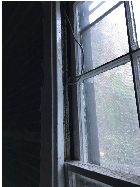
POSSIBLE ORIGINAL SASH AND FRAME IN DISREPAIR
