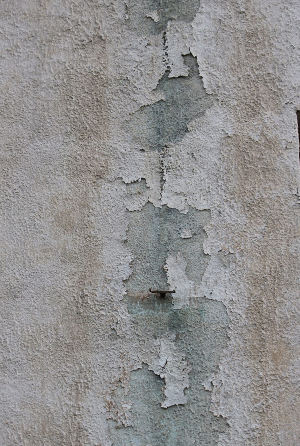
Stucco Conditions: Evidence of Previous Coating
