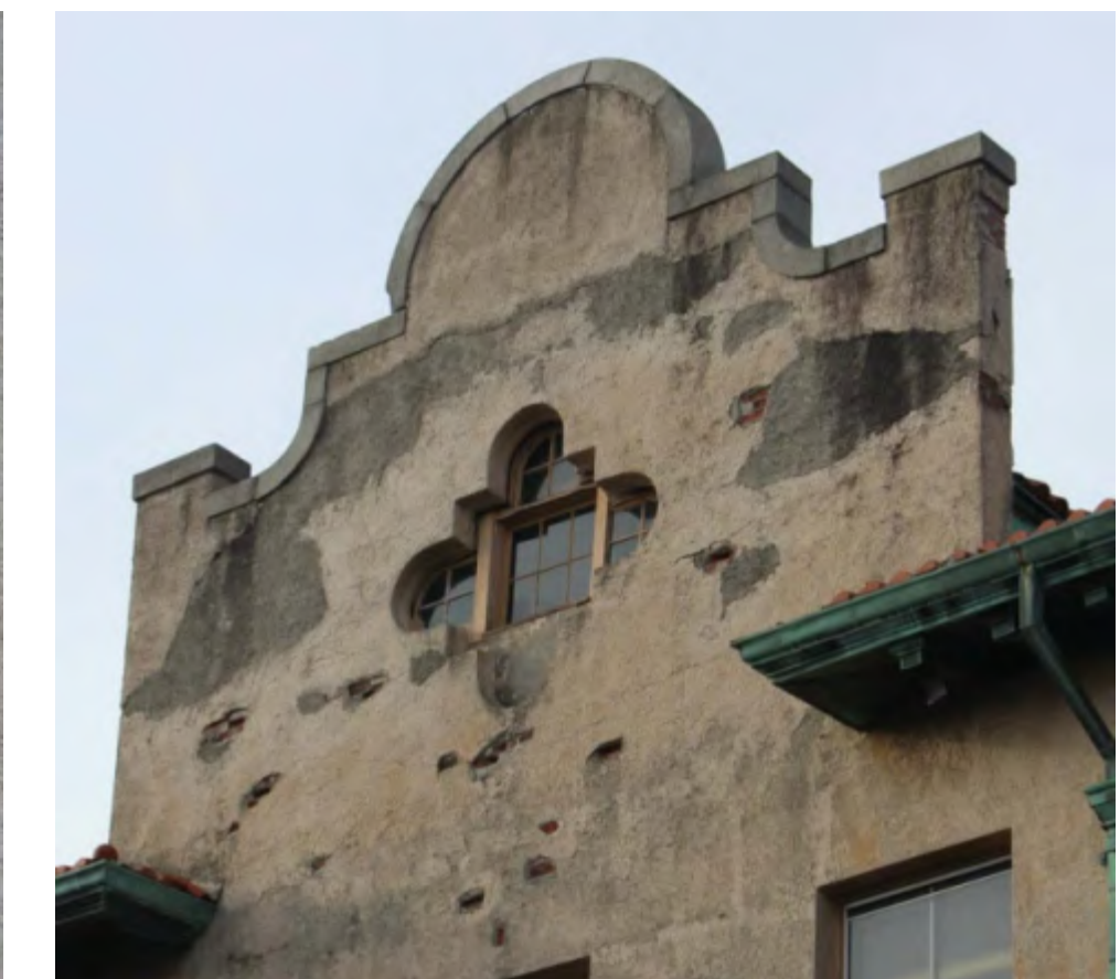
STUCCO HAS AREAS OF WATER DAMAGE AND MISSING MATERIAL, BUT GENERALLY SOUND.
