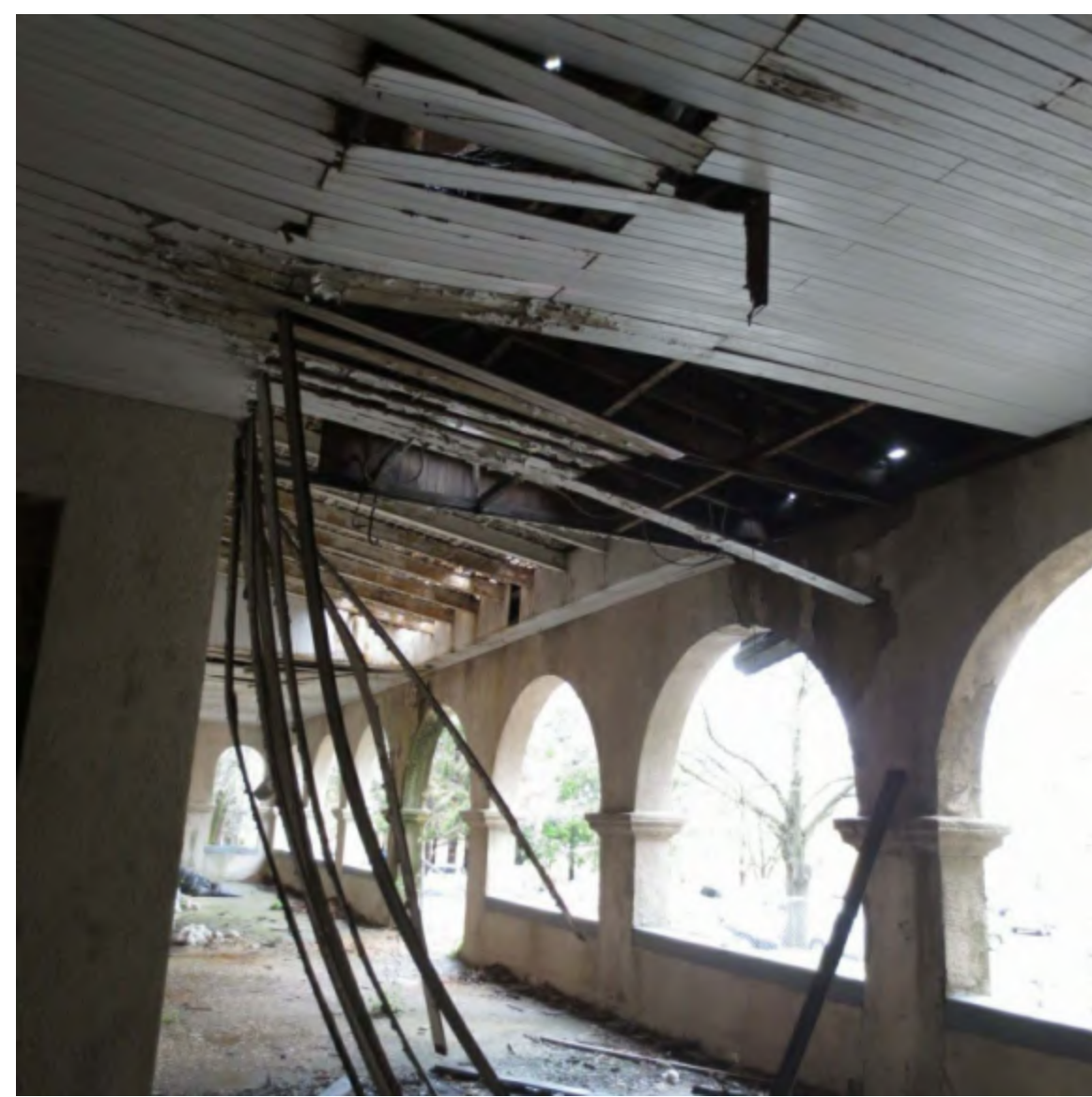
DAMAGED WOOD CEILING AT NORTH PORCH
