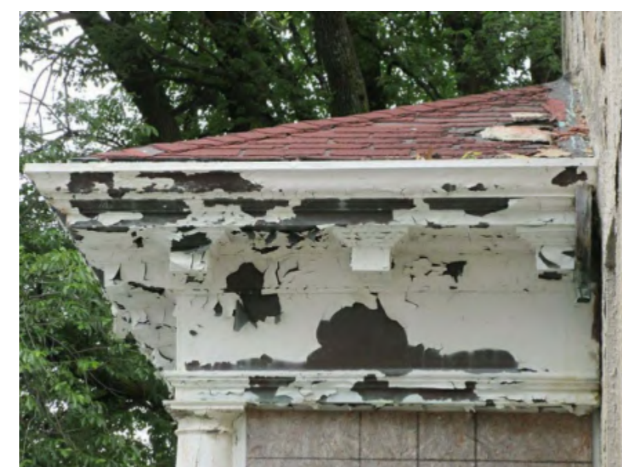
TYPICAL METAL CORNICE WITH PEELING PAINT AT COURTYARD ENTRY PORTICO AND ROOF
