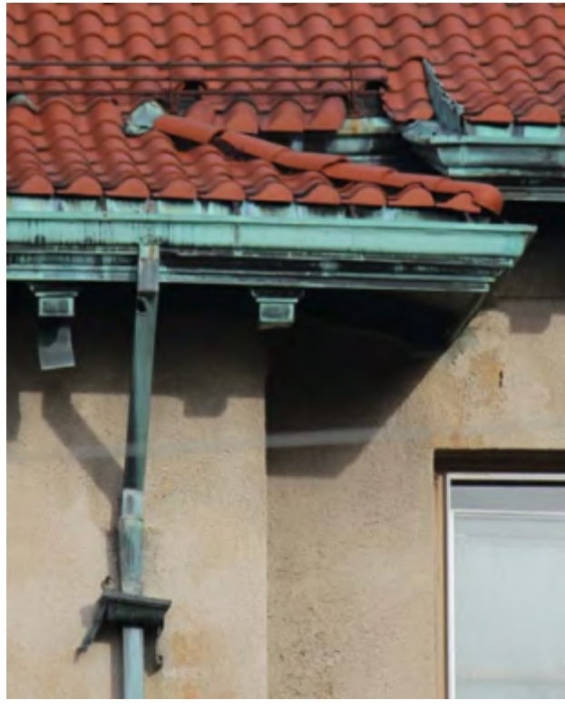
EXISTING COPPER DOWNSPOUTS ARE MISSING OR DAMAGED AT SOME LOCATIONS
