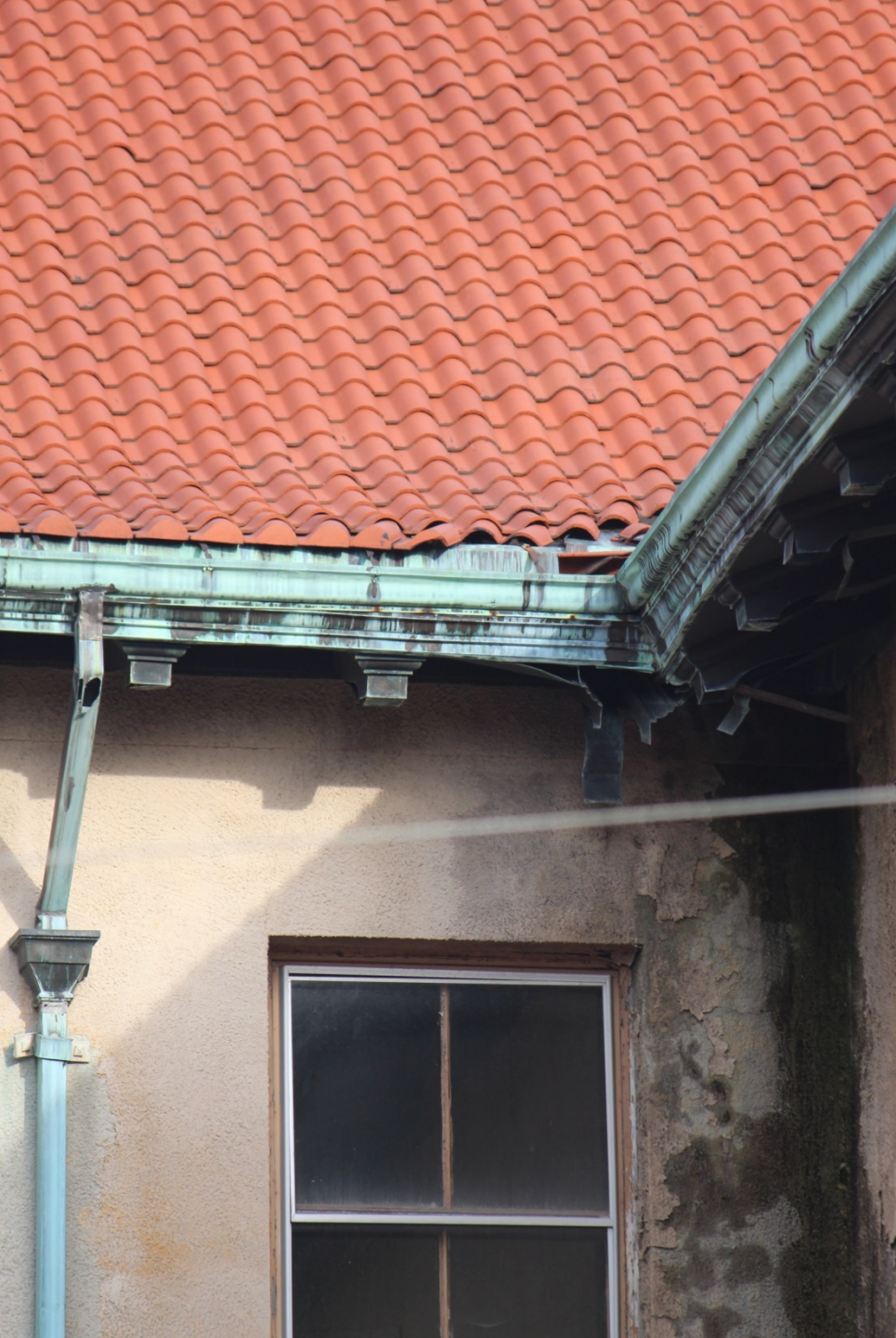
East (entry) Façade with necessary cornice repair due to water damage. Roof Repair to utilize salvaged material from nurse's wing. Water damage has manifested itself inside of building.
