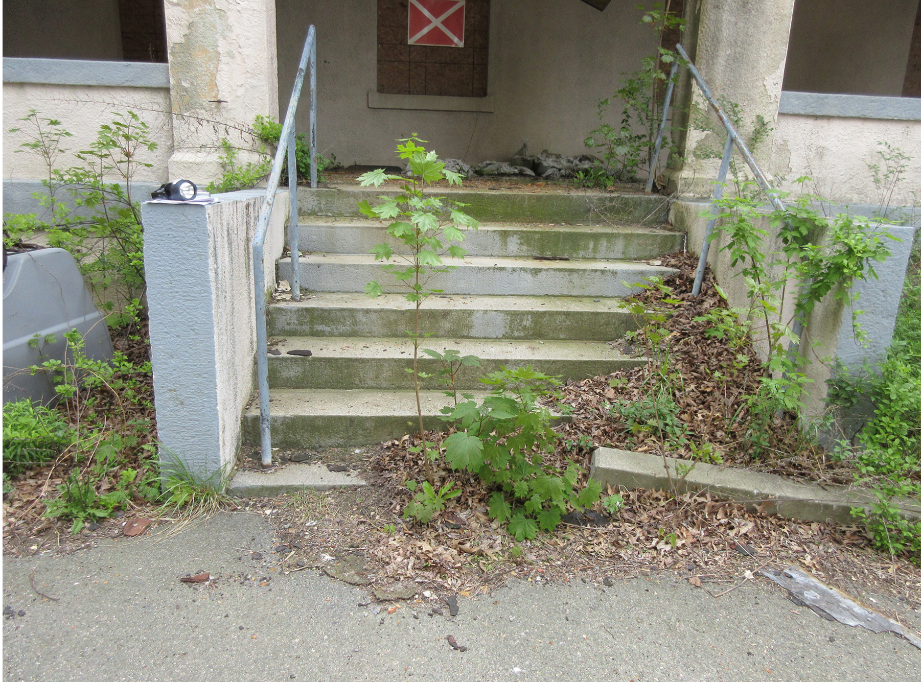
North porch is not currently accessible and will be made accessible with new ramp concealed in porch
