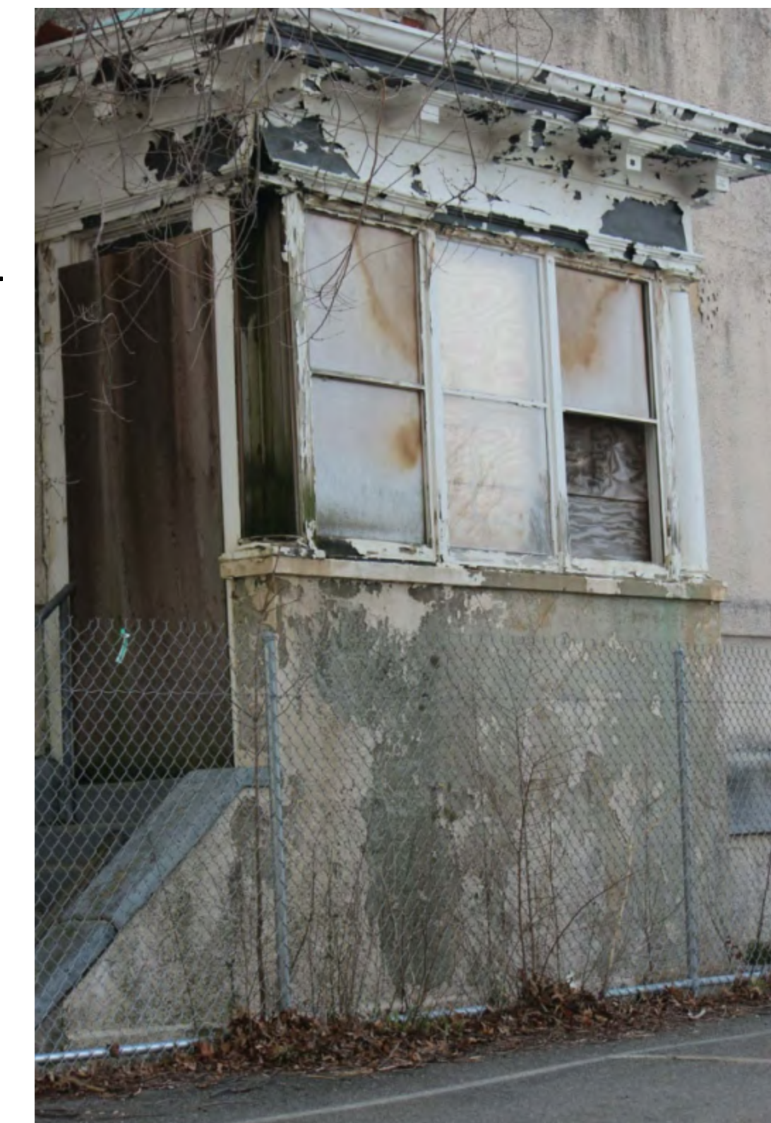
SMALL ENTRIES WERE ORIGINALLY OPEN PORCHES, AT SOME POINT ENCLOSED WITH WINDOWS AND DOORS.
