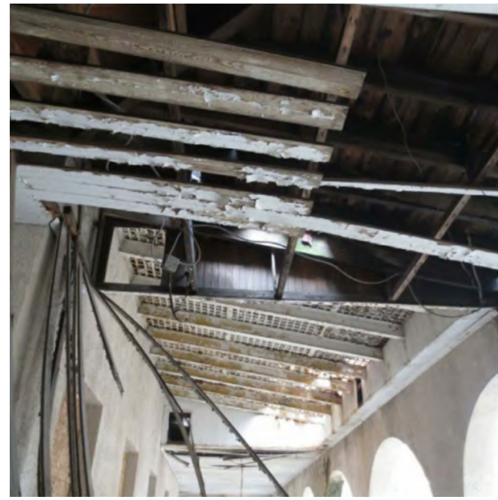
DETAIL VIEW OF DAMAGED CEILING, SHOWING WOOD AND METAL FRAMING (ORIGINAL SKYLIGHT?).
