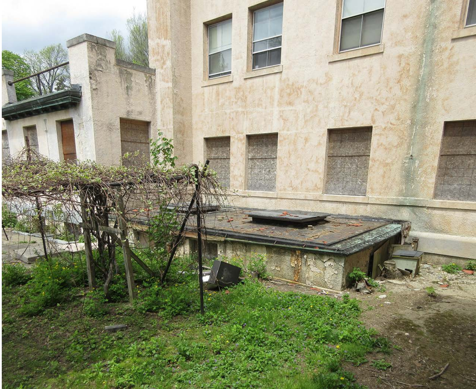
Existing light well is structurally unsound and is being removed to enable an accessible ramp to be installed to basement level where pet wash, boiler storage and maker space is located.
