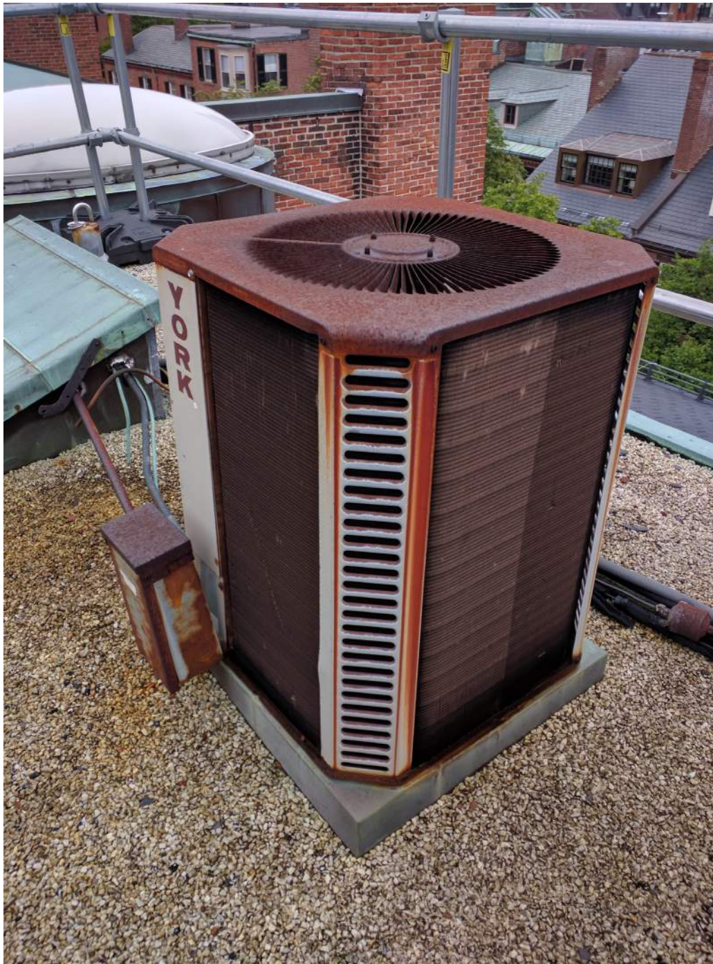
EXISTING RTU TO BE REMOVED
