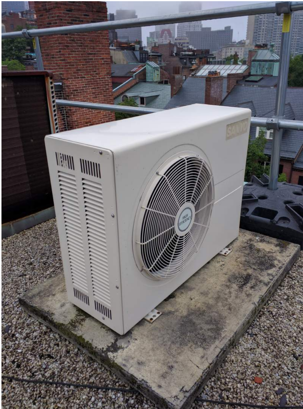
EXISTING RTU TO BE REMOVED
