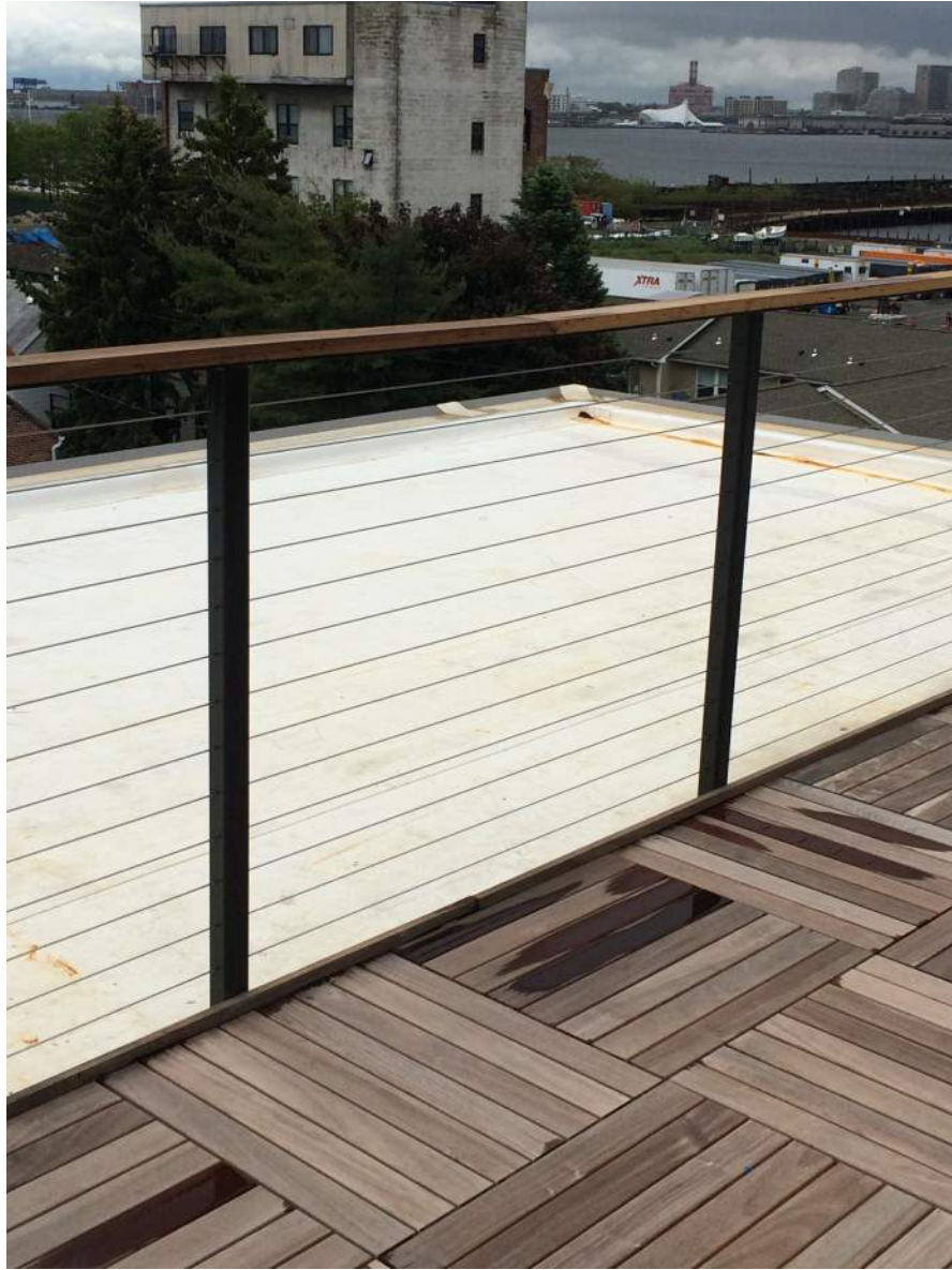
PHOTOGRAPH OF SIMILAR INSTALLATION
