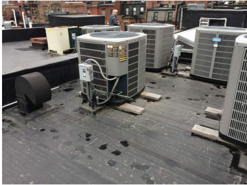
EXISTING ROOF TOP EQUIPMENT
