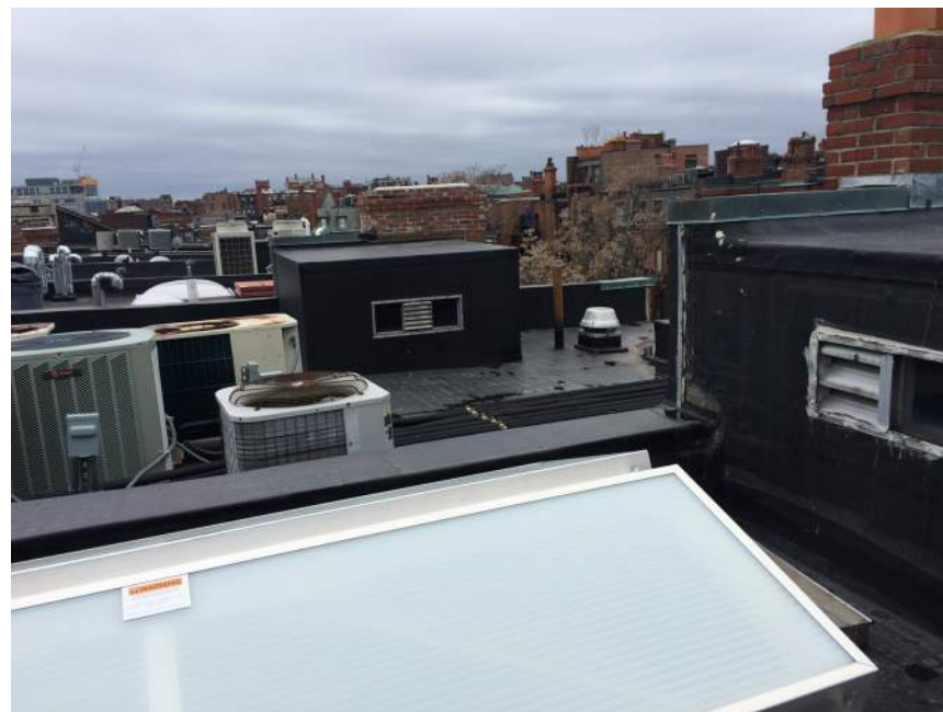
EXISTING ROOF TOP EQUIPMENT
