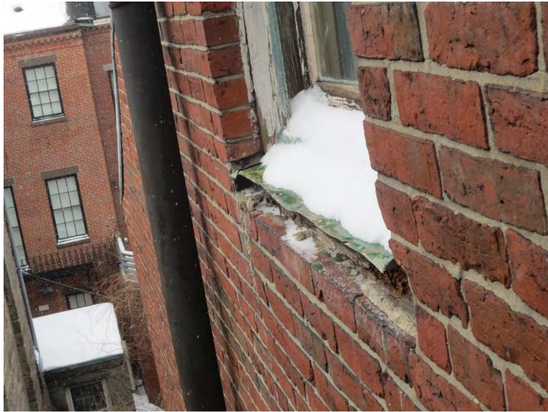
Wood Sill at Fifth Floor Side Window (505)
