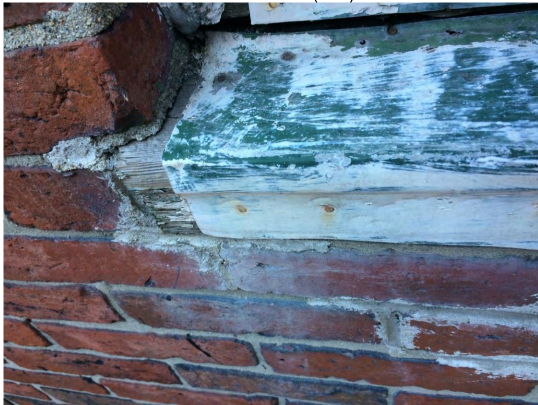
Wood Sill at Fifth Floor Side Window (504)
