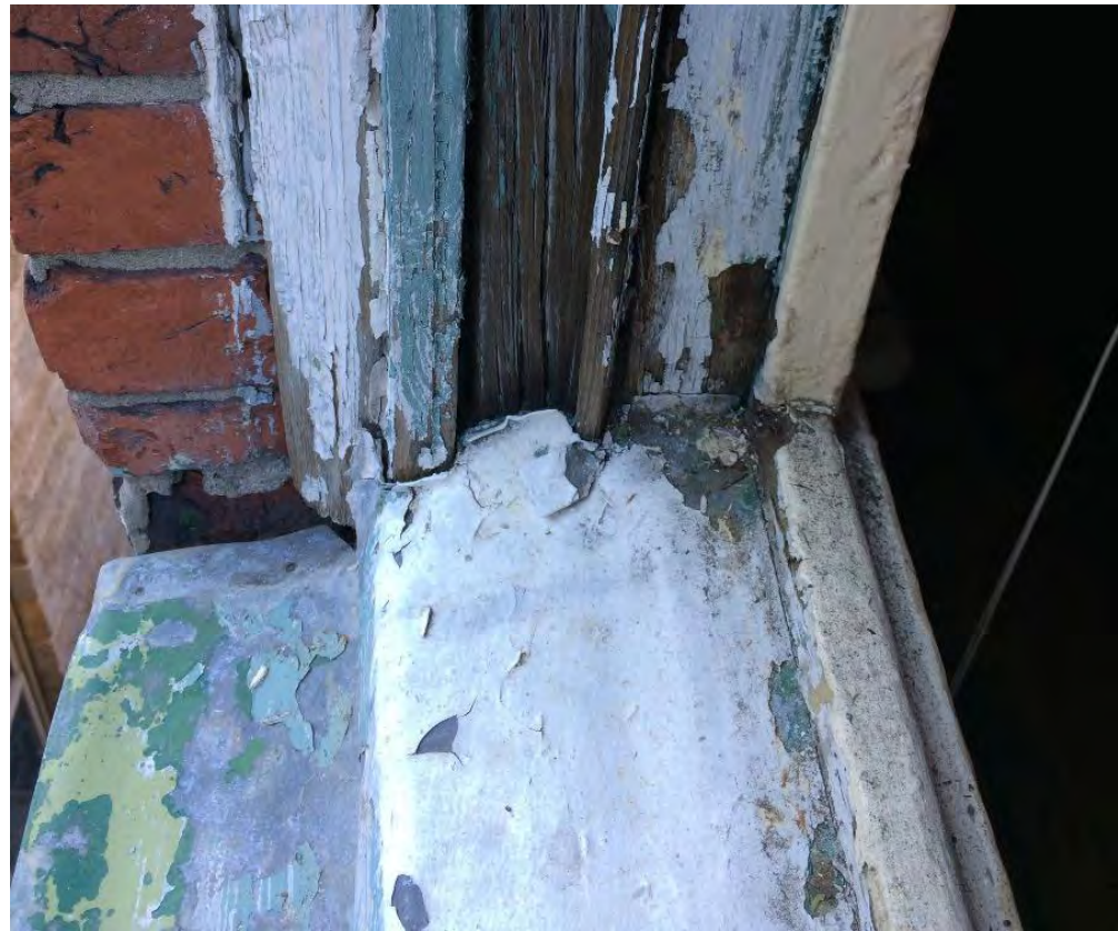
Wood Sill at Fifth Floor Side Window (505)
