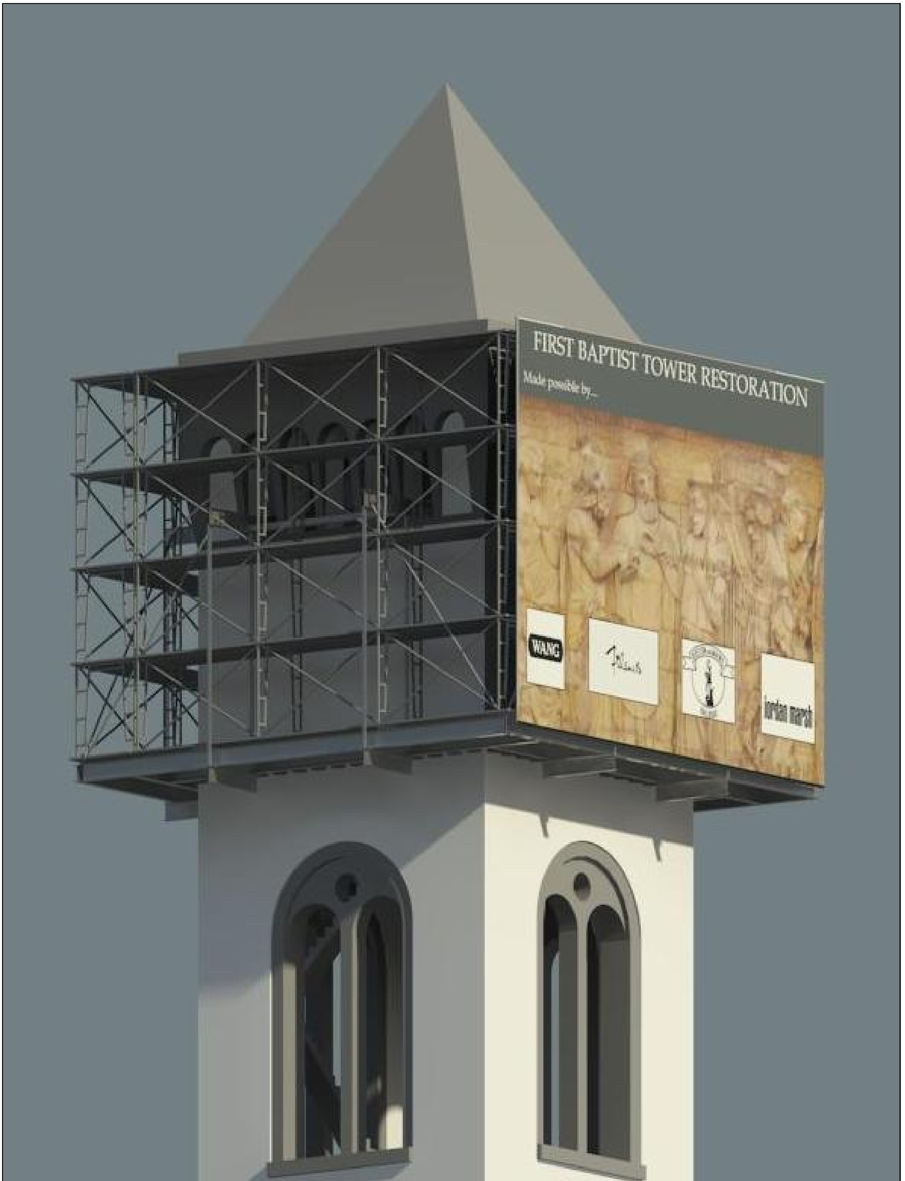
SCRIM IN RELATION TO WORKING PLATFORM (Scrim will actually be on all four sides)
