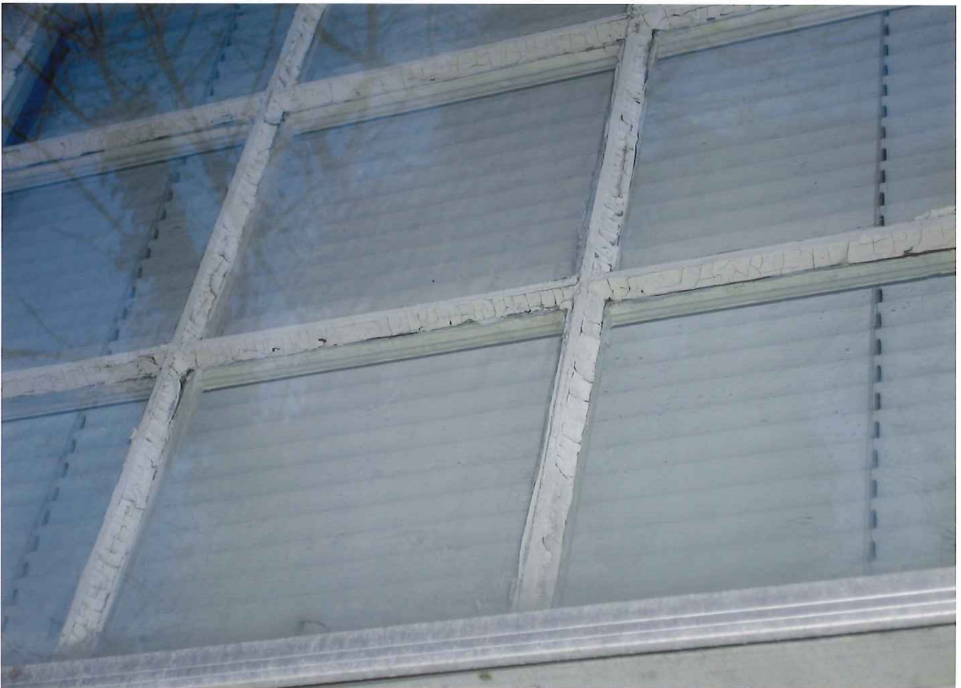
DETERIORATED PUTTY ALL OVER
