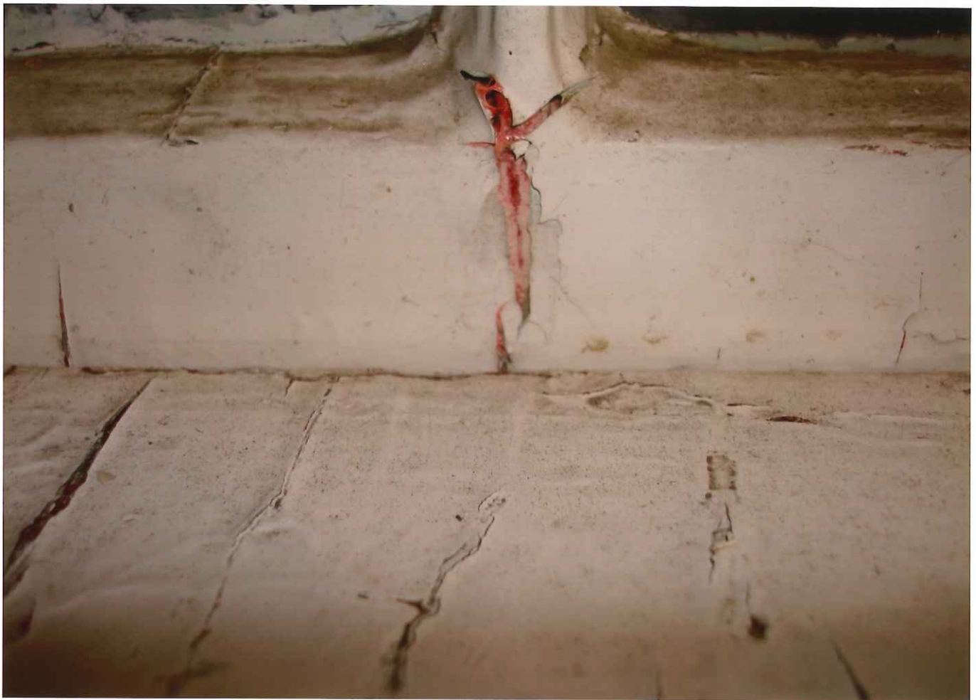
MANY LAYERS OF LEAD PAINT CRACKING
