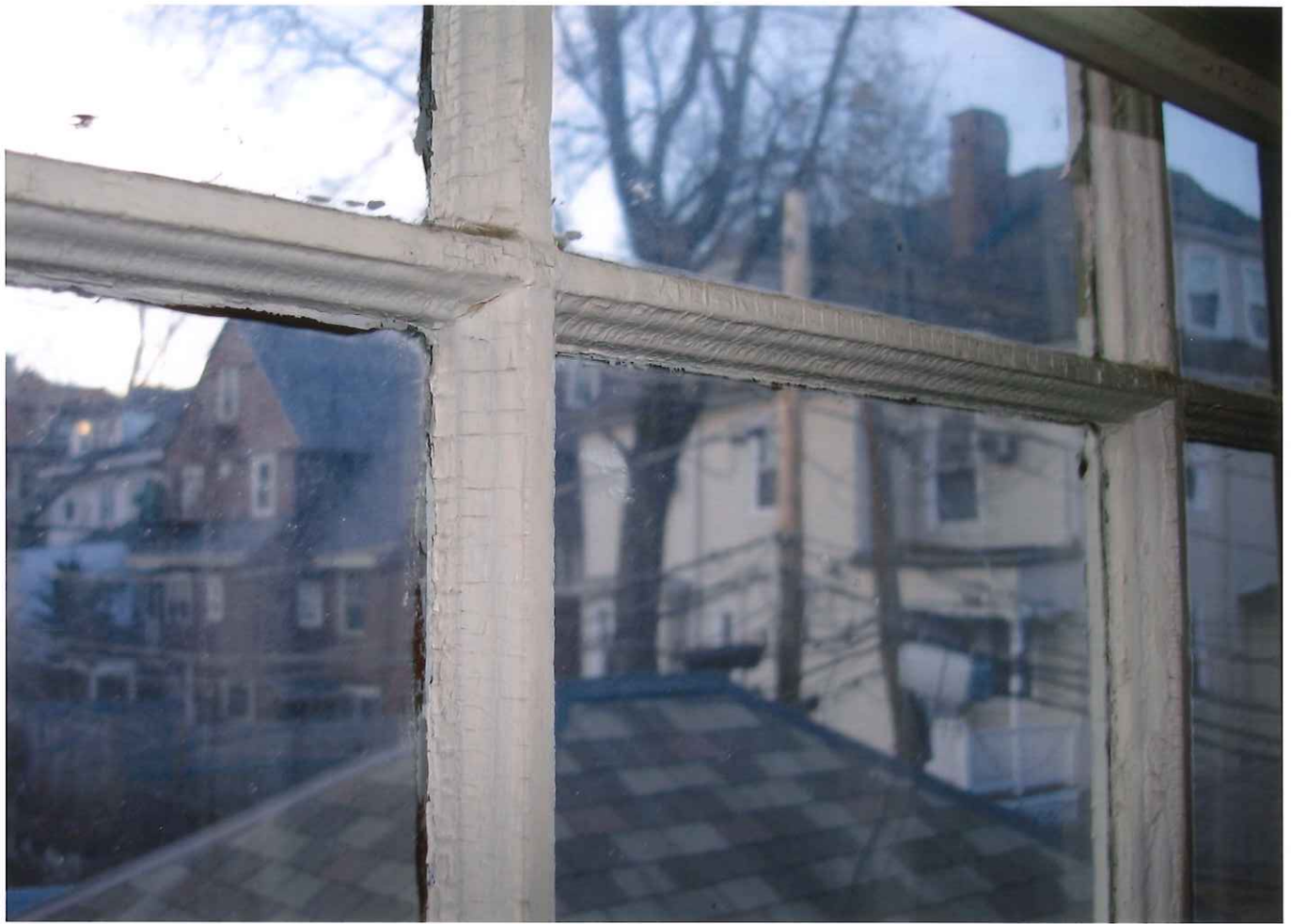
LEAD PAINT EVERYWHERE
