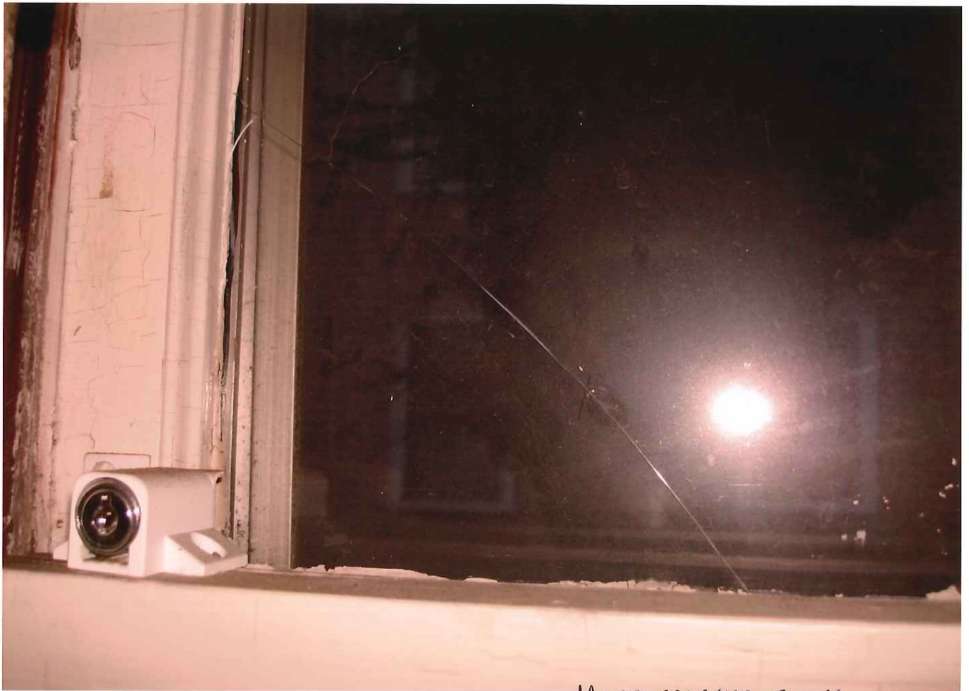
MORE CRACKED GLASS
