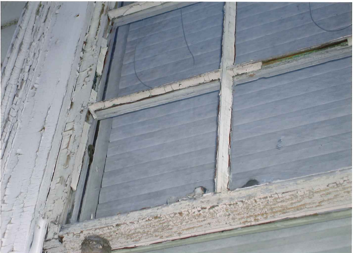
DETERIORATION AND MISSING MUNTIN
