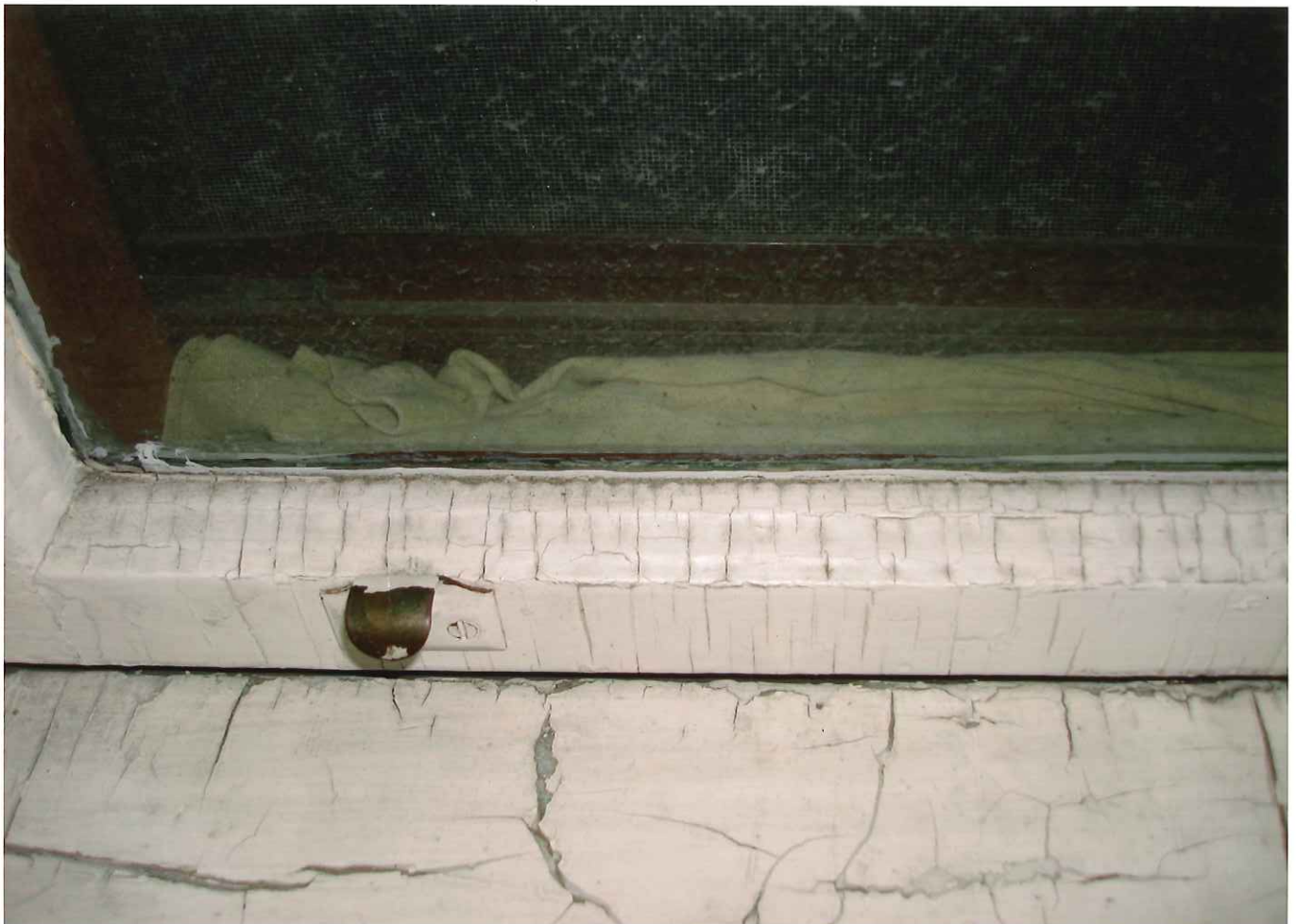
CRACKED LEAD PAINT AND WINDOW DOES NOT CLOSE
