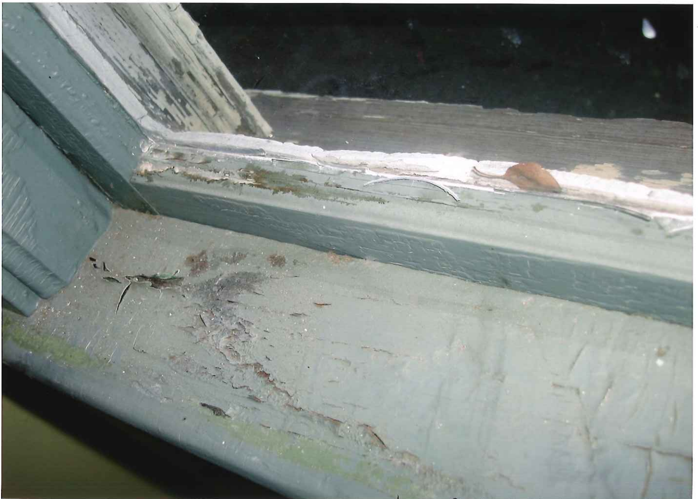
LEAD PAINT & MISSING PUTTY
