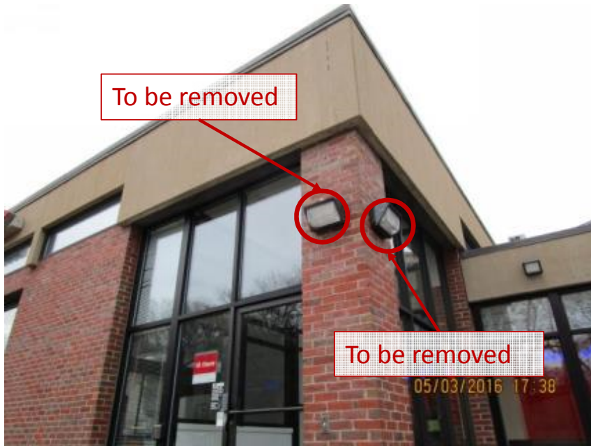
Wall lights – right front corner May 3, 2016
