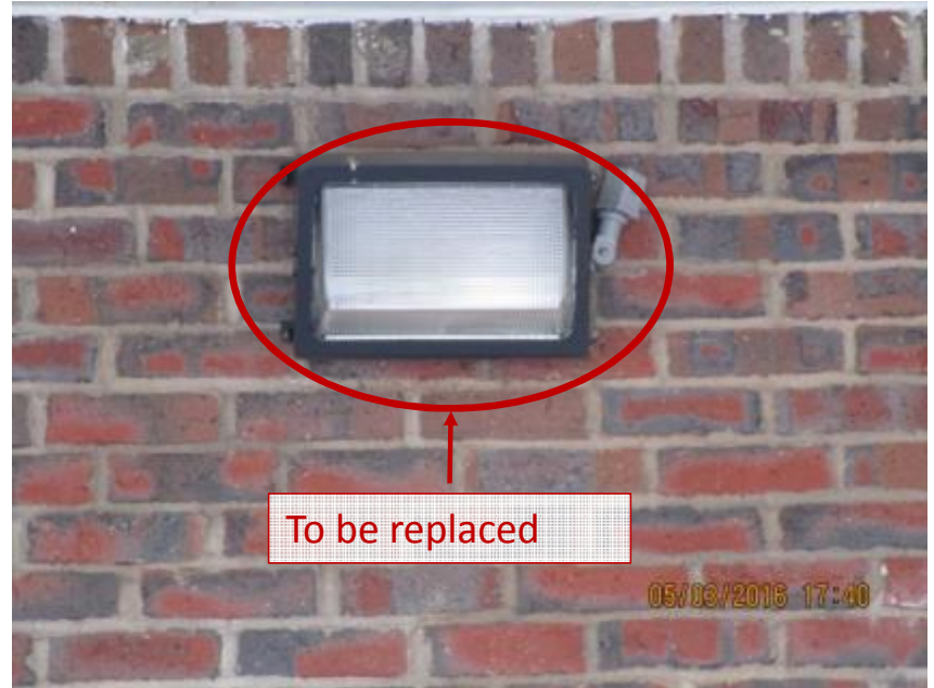
Wall light - rear May 3, 2016
