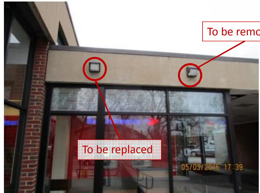
Wall light – right front corner May 3, 2016
