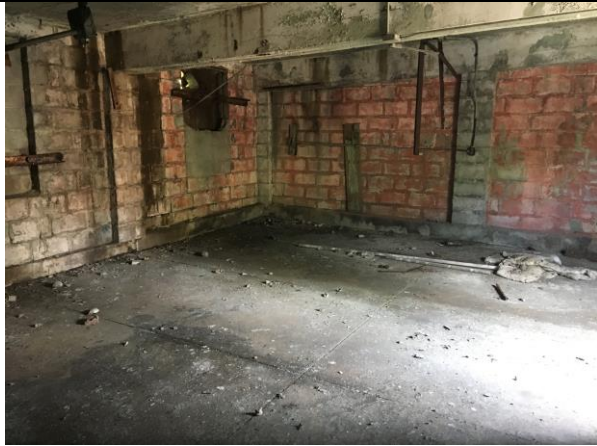
Photo 15: View of the interior of the garage on Site No. 12. Minimal black staining is visible.
