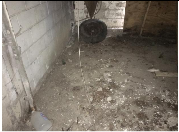
Photo 14: View of the interior of the garage on Site No. 12. Minimal staining and paint chips on the floor.
