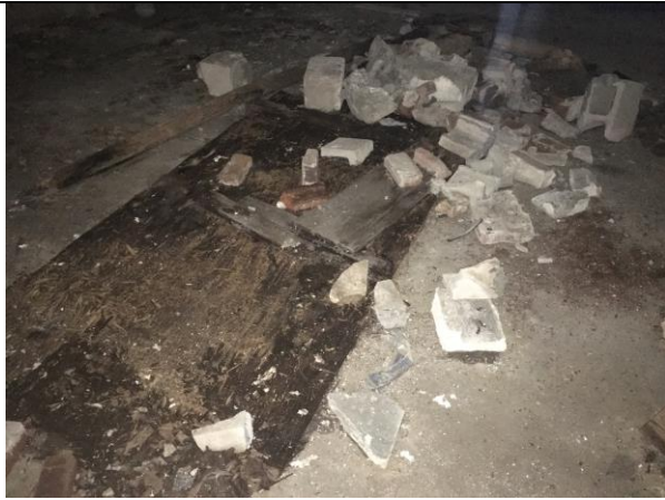
Photo 13: View of the interior of the garage on Site No. 12. Portion of the roof is caving in.
